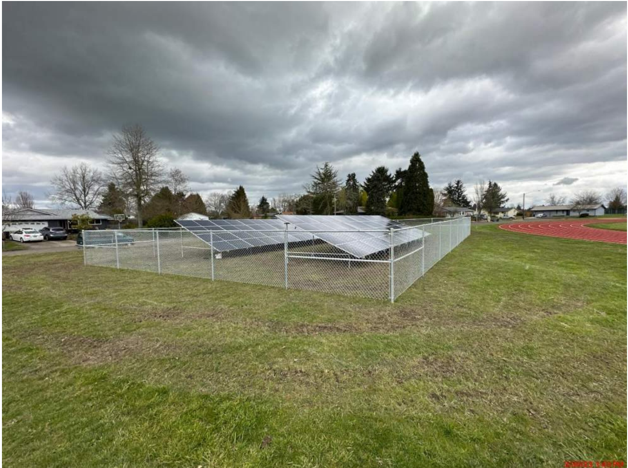
Cheldelin – New solar installation
