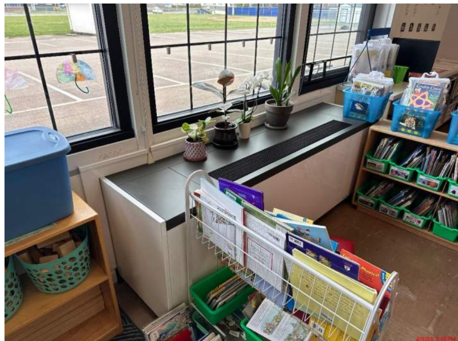
Franklin – New unit ventilator in place
