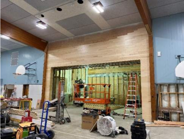
Gym – Stage Opening
