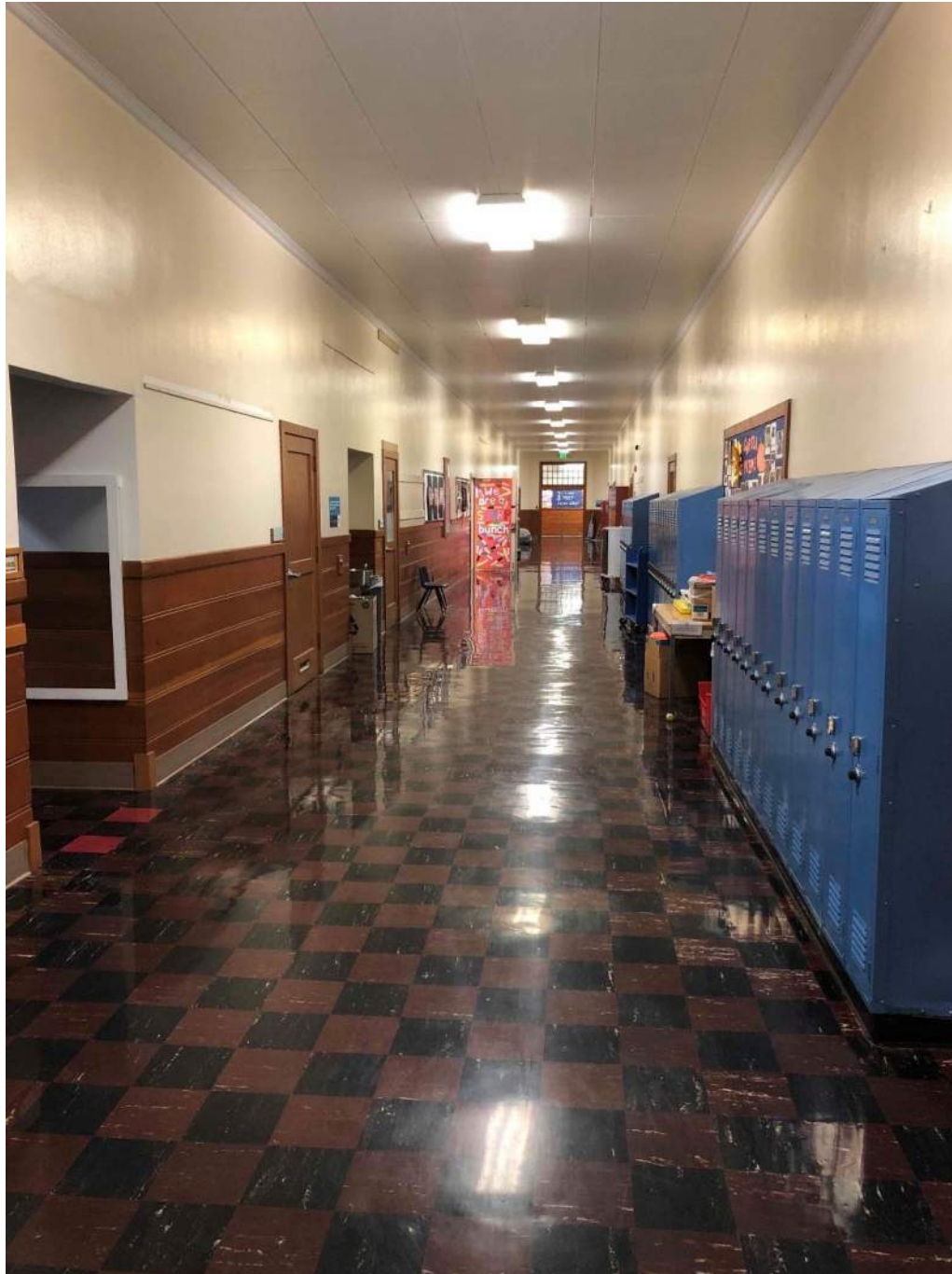
Franklin Hallway – flooring to be abated
