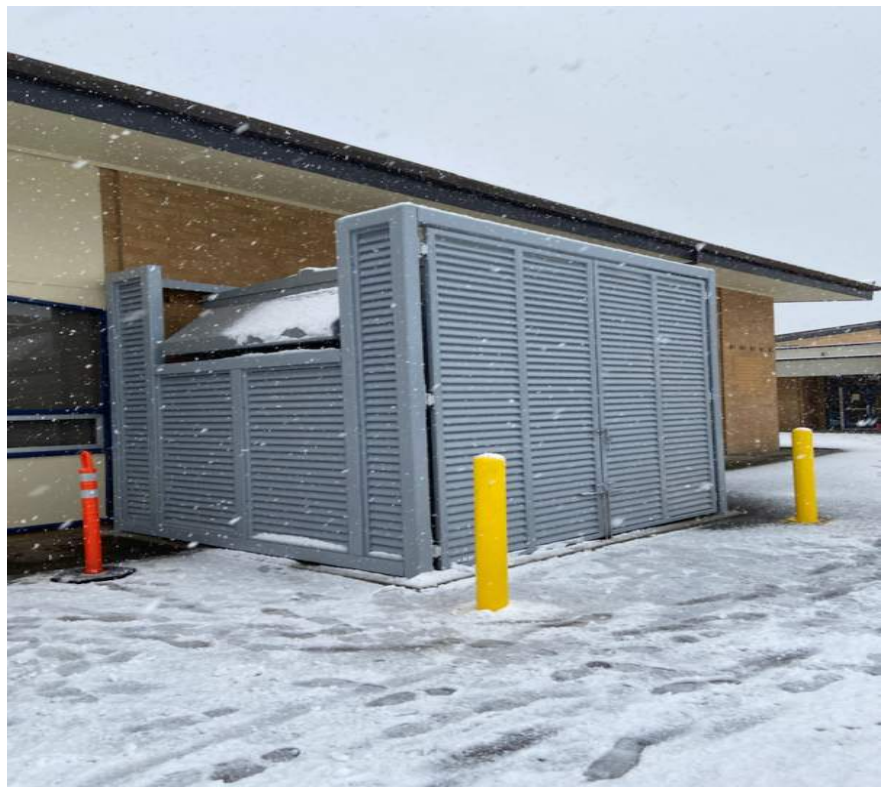
New HVAC enclosure outside STEAM
