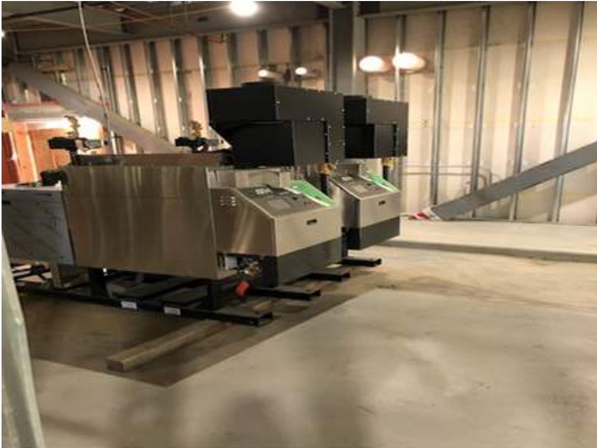
Mechanical equipment awaiting installation
