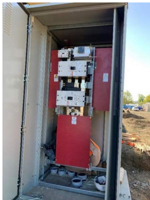
New electrical switchgear set
