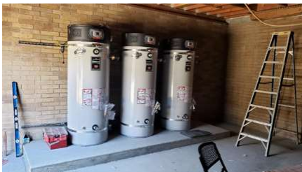
New hot water heaters installed in Building A Boiler room
