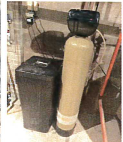
Building Water Softener
