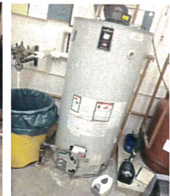
Kitchen Water Heater
