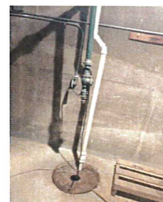
Basement Sump Pump
