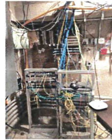
Lower Level Data Room
