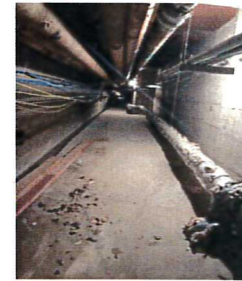
Water Piping at Tunnels
