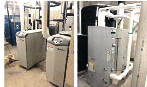
HS Water Heaters
