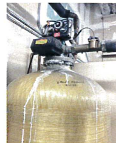
HS Water Softener
