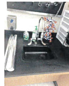
Science Room Sink
