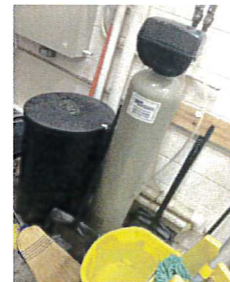
Kitchen Water Softener
