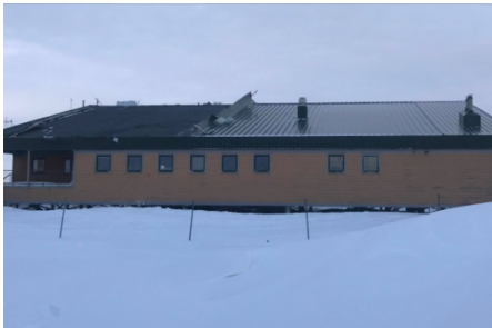
937 938 Wales roof damage
