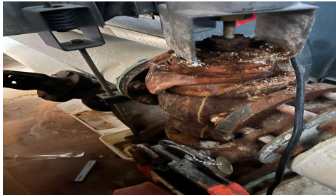
Chiller valve needing replacement at Rupert Elementary
