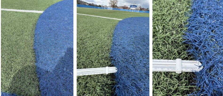
Seam separation on log to be a 1 inch wide gap
