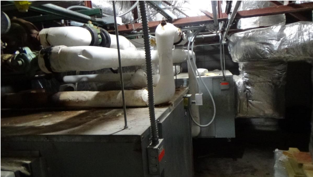
Band & Chorus Penthouse Mechanical Room
