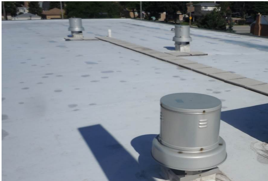
19. NW Roof Exhaust Fans, circa 1997
