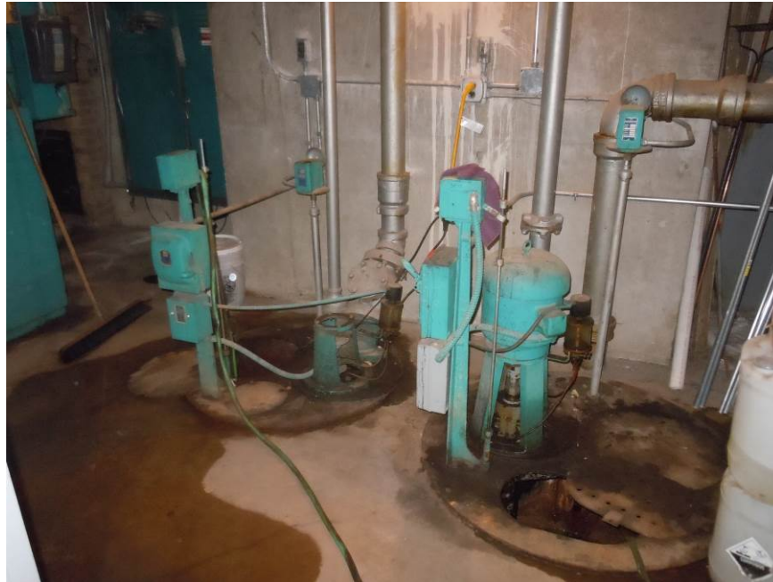
34. 1963 Sump Pump and Sewage Ejector
