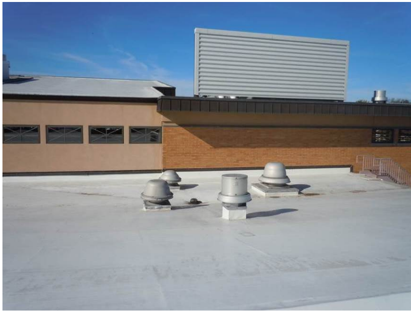
20. East Roof Exhaust Fans, included 1963 Fans
