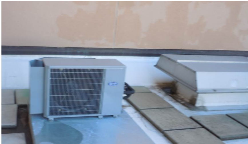
14. 2013 IT Closet AC Condensing Unit CU2 and Lower Level Smoke Relief Intake – Lower W Roof
