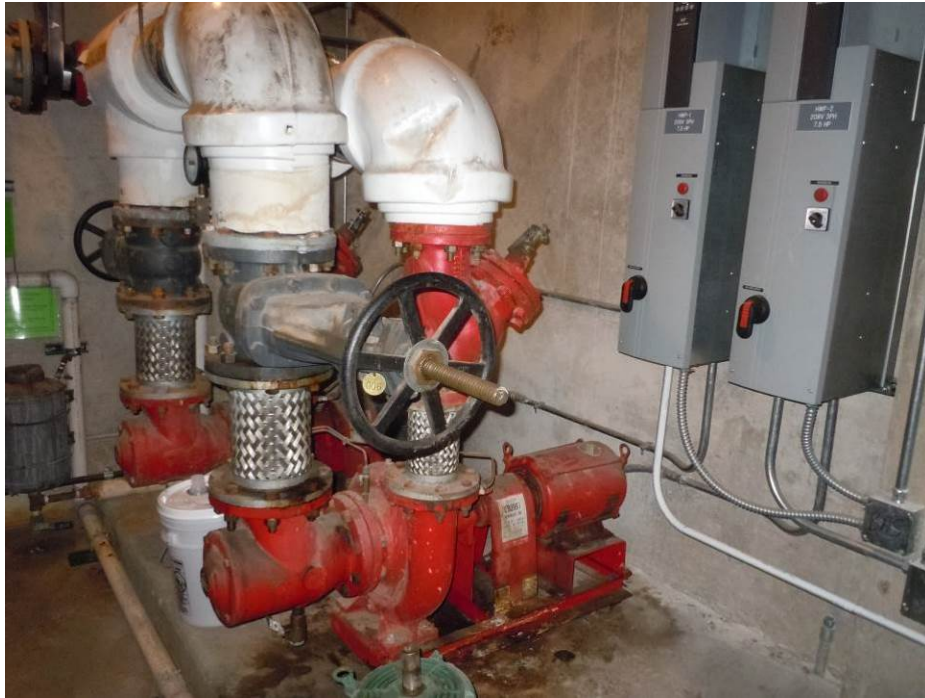
3. 1997 Hot Water Heating Pumps with new variable Frequency Drive (VFD) control
