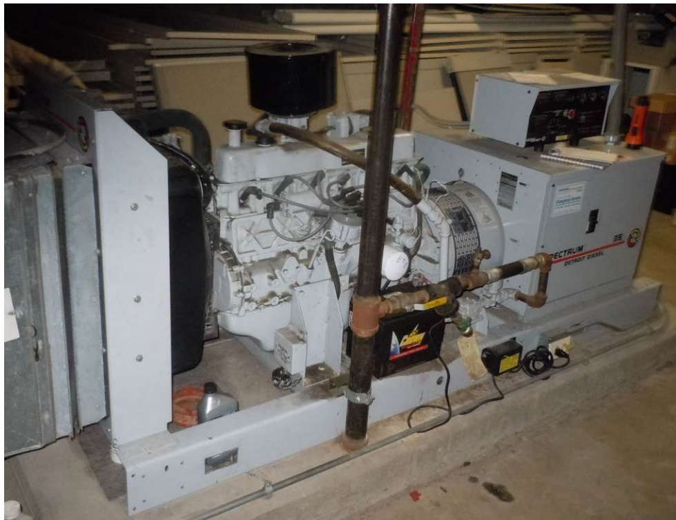
27. Emergency Generator in Center Basement, 1997 Installation
