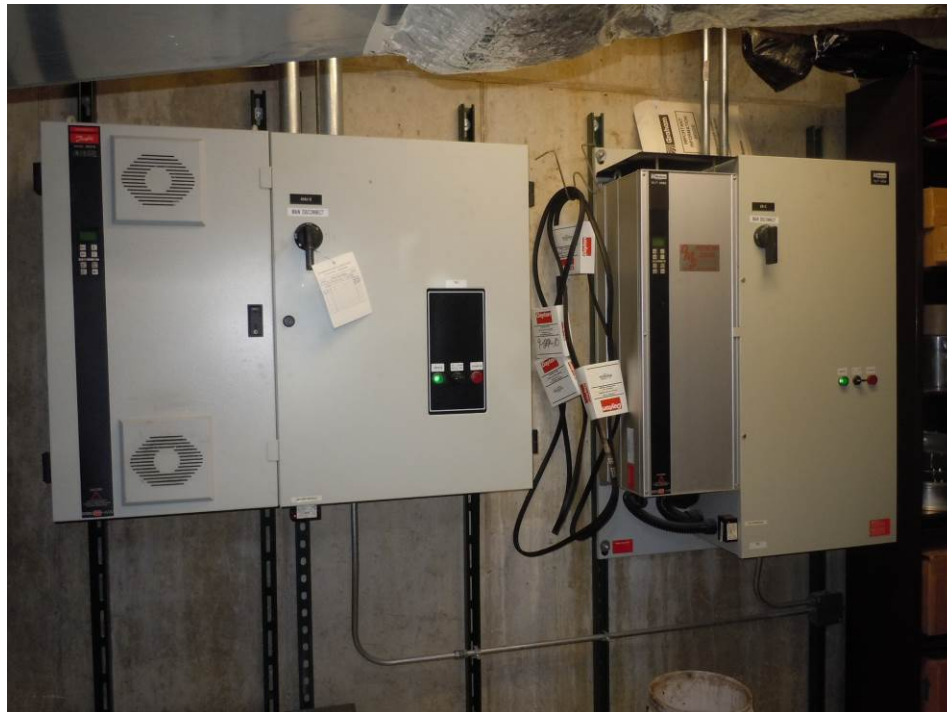
13. 1997 Variable Air Drive for AHU-2 and ER-2
