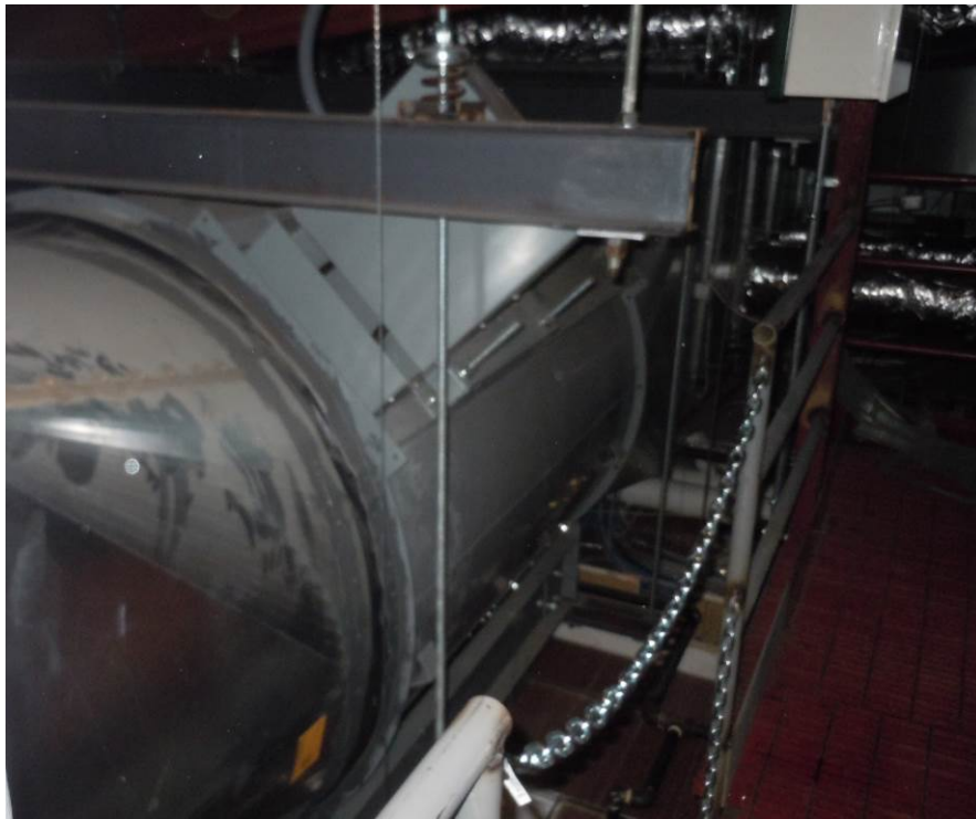
10. 2013 Exhaust Return Fan 1 in Northeast Attic
