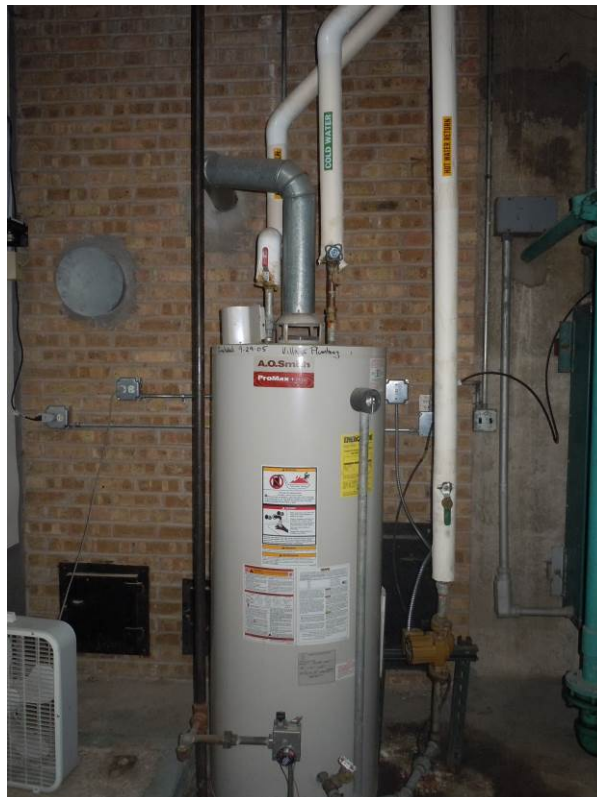
35. 2005 Domestic Water Heater
