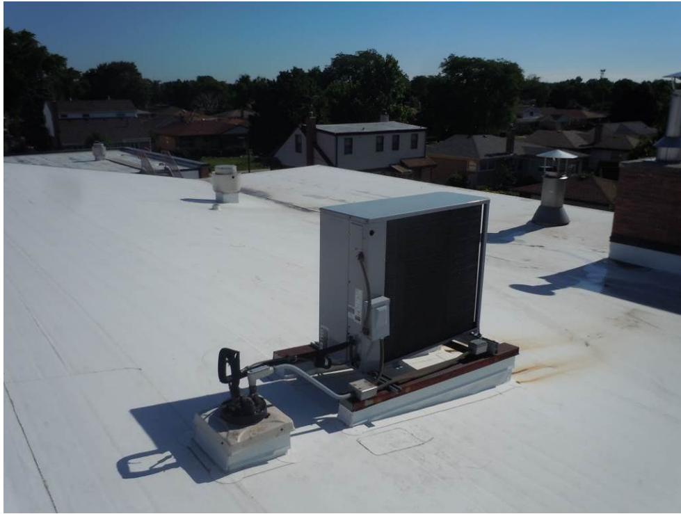
16. 2010 Roof-mounted IT Room AC Condensing Unit
