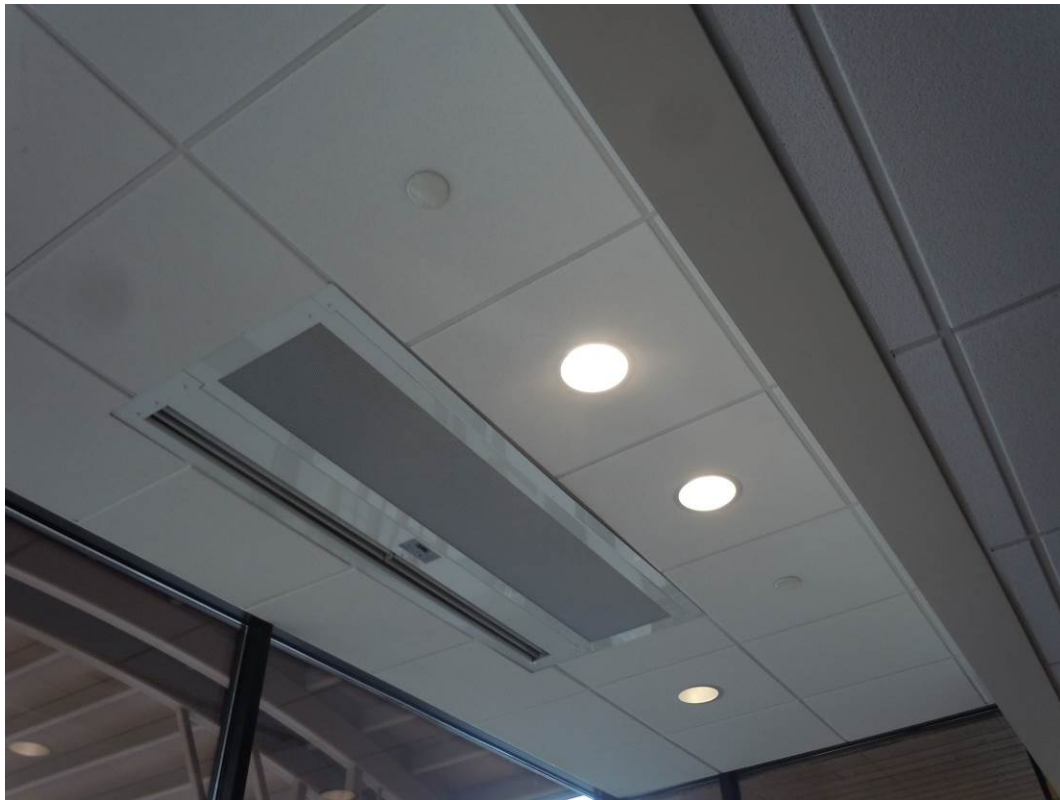
23. Door Heater, West Main Entry
