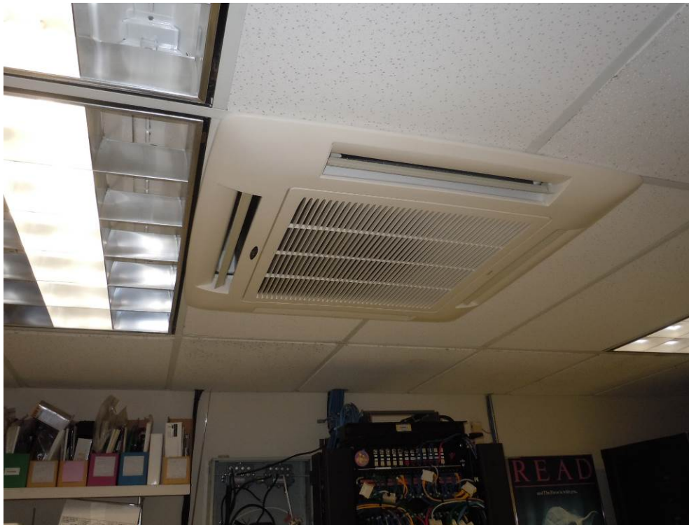
17. IT Room Air Conditioner Fan Coil Unit
