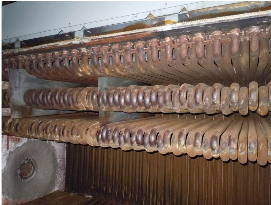
2. 1997 Heating Boiler (bent water tubes during 2011 summer service, 2 nd photo)
