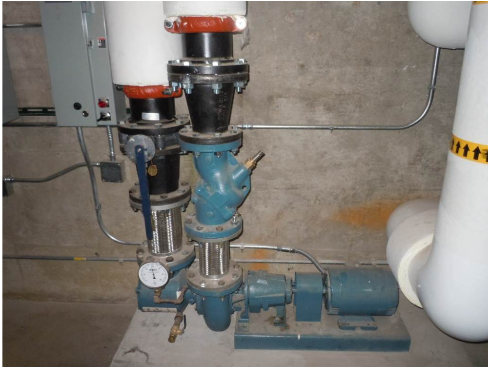
5. 2013 Hot Water Heating Pump
