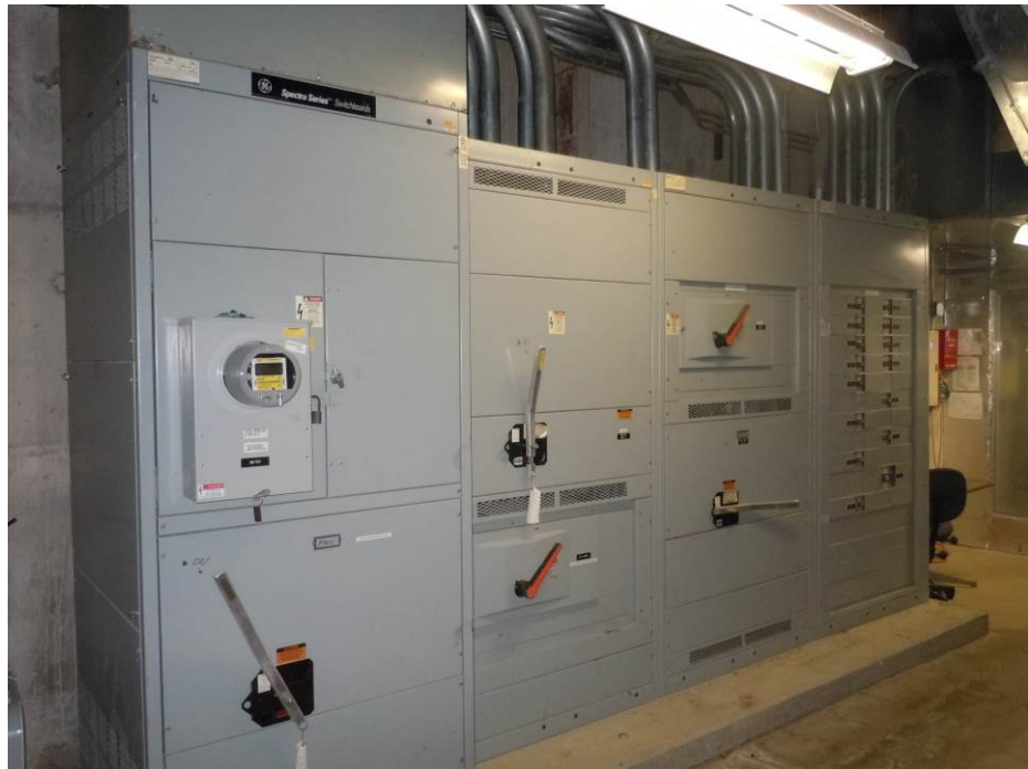
26. Electrical Service Switchboard, circa 1997
