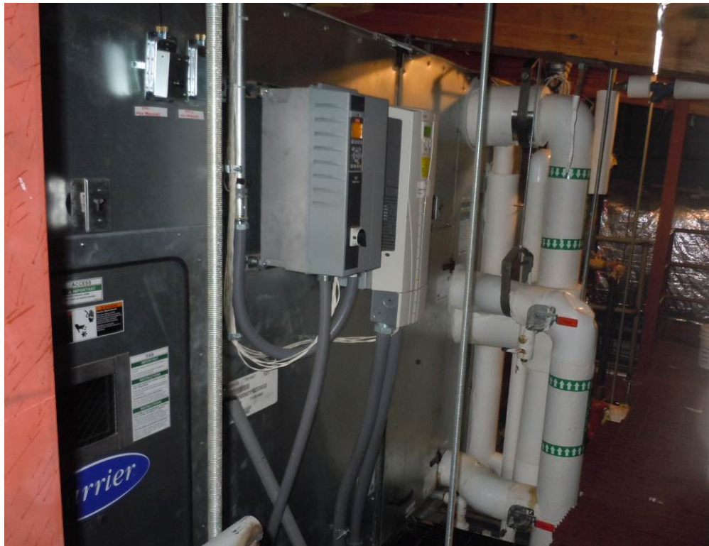
9. 2013 Air Handling Unit AHU-1 with HW and CHW Piping
