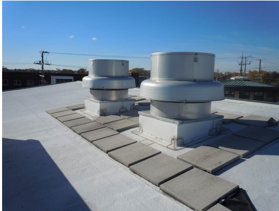
18. Center Roof Smoke Relief Fans
