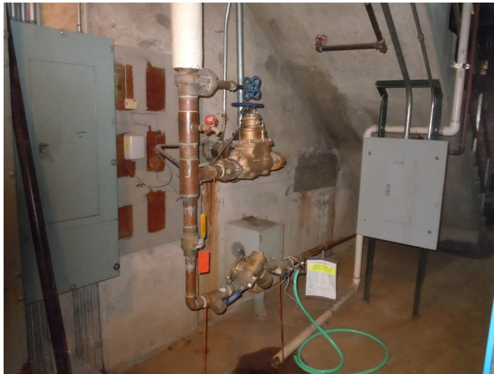
31. Domestic Water Service in East Basement
