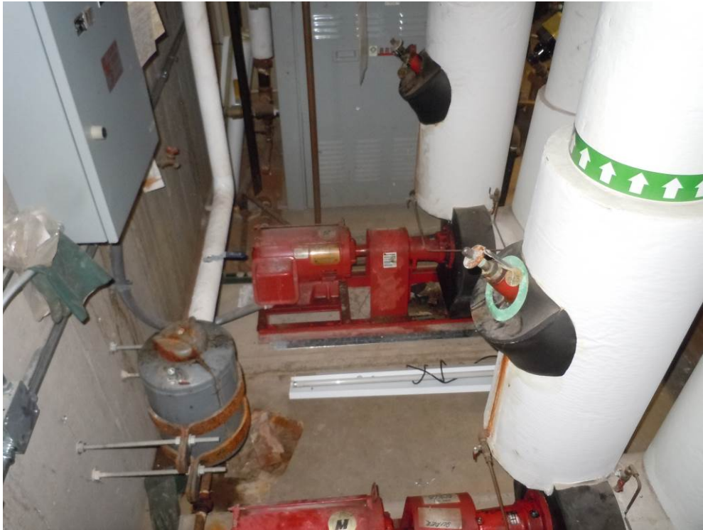
7. Air Conditioning Chilled Water Pumps, 1997
