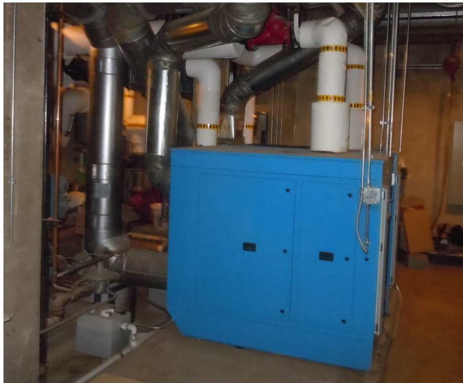
1. 2013 Heating Boilers, 90 Percent Thermal Efficient
