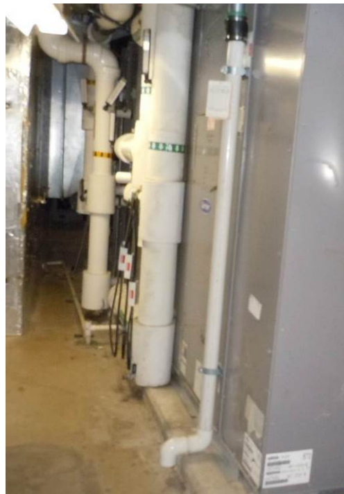
11. 1997 Air Handling Unit AHU-2, Partial View with HW & CHW Piping
