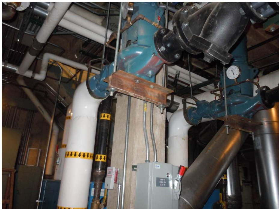
4. 2013 Boiler Hot Water Pumps
