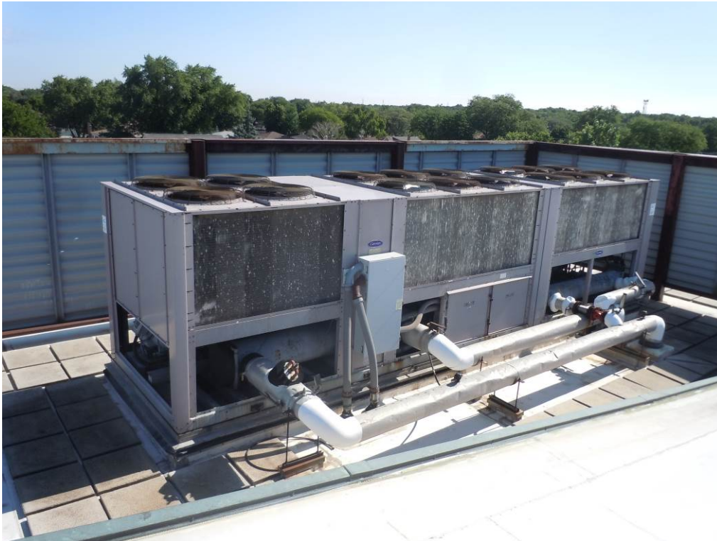
6. Roof-mounted Air Conditioning Chiller, Circa 1997
