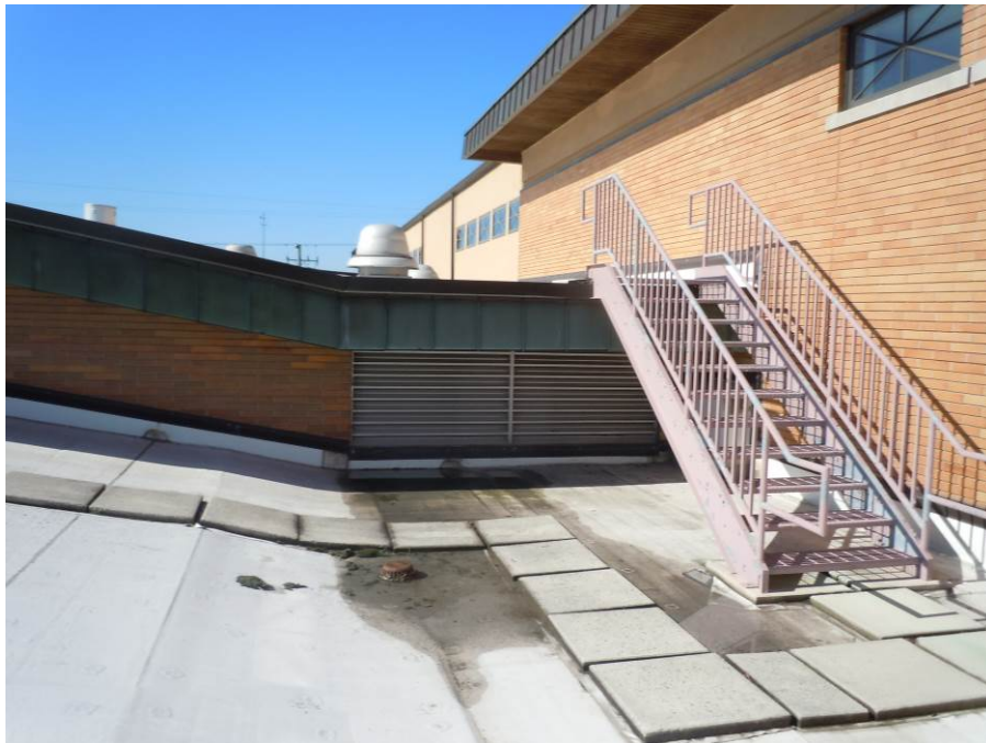
22. East Roof looking South, with AHU-1 outside air louver, exhaust fans
