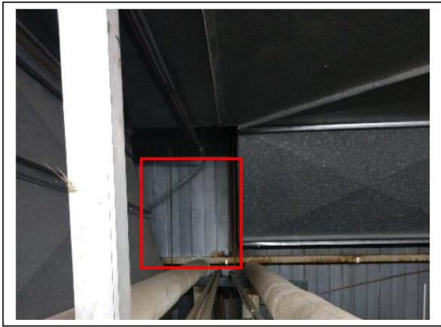
Photo # 5 Rooftop Penthouse White Caulk between Penthouse Walls (Every 2' to 3') Positive for Asbestos
