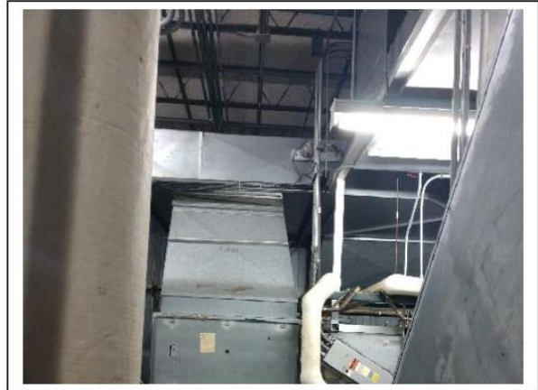
Photo # 2 Rooftop Penthouse Mud Joint Fittings on Fiberglass Lines Negative for Asbestos
