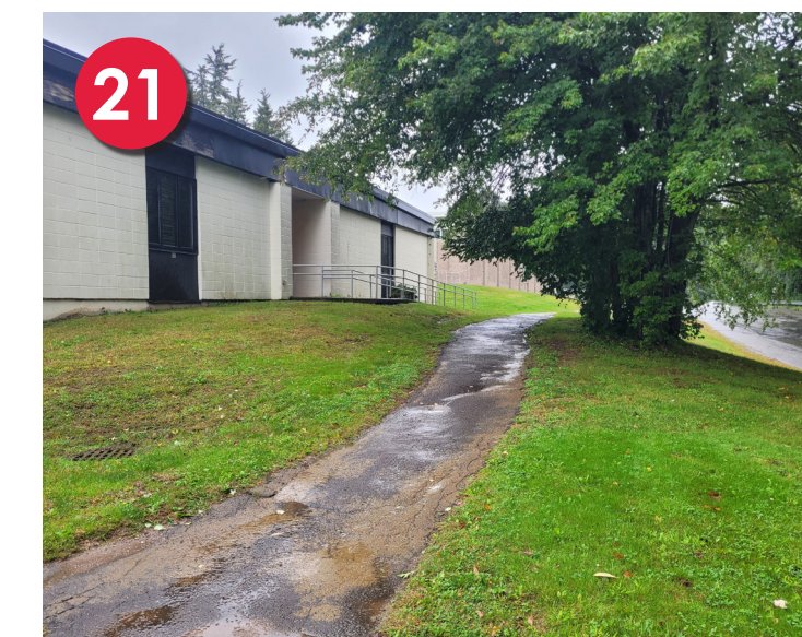
Biofiltration Swales Drainage Area 4
