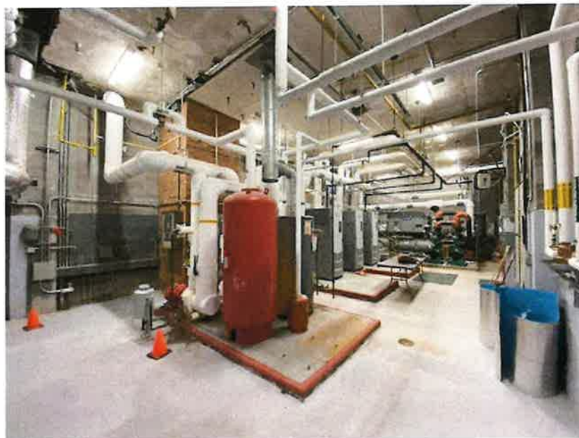
Boiler & Chiller plant feeding 2-pipe system
