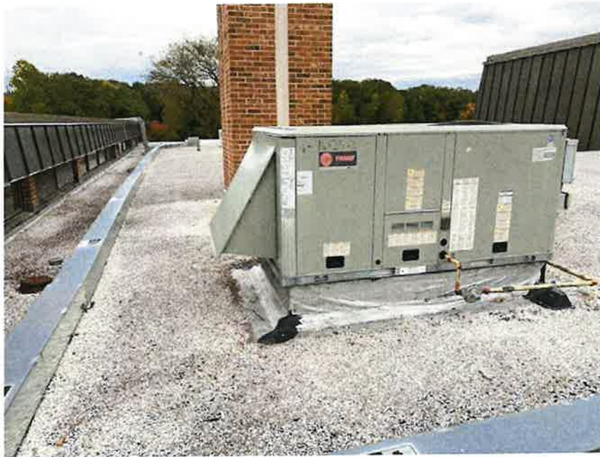
Packaged rooftop unit serving Office area
