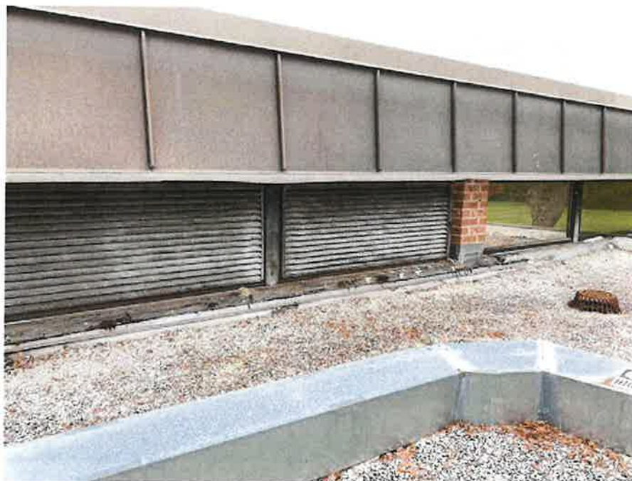
Typical fresh air louver serving Unit Ventilators
