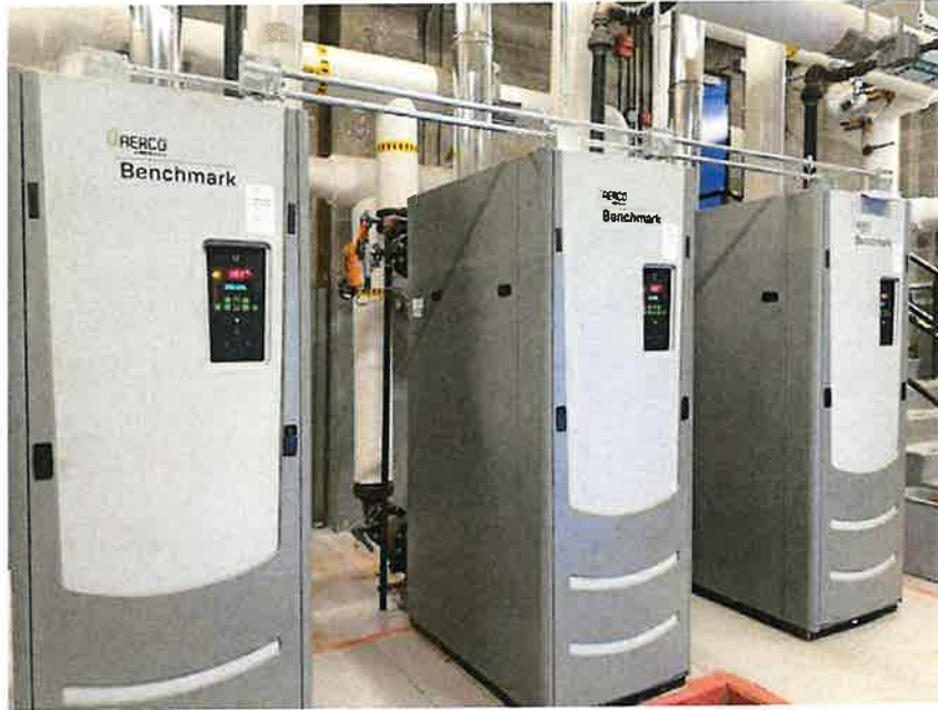
Condensing boilers - recently replaced
