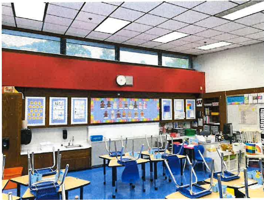
Typical Classroom showing Unit Ventilator
