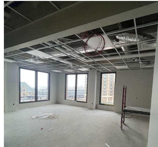
2 nd Floor Lighting & HVAC
