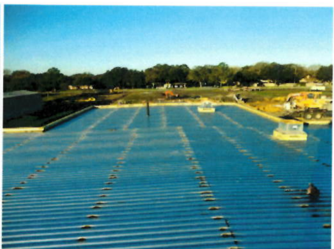
6. Mechanical roof curbs
