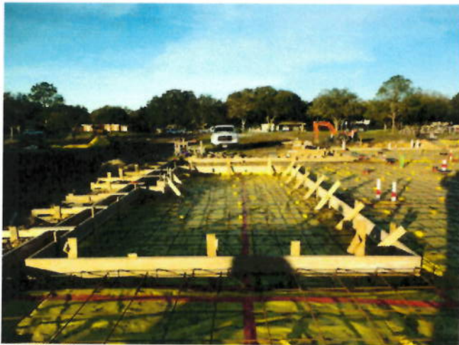
3. Walk in cooler / freezer slab depression
