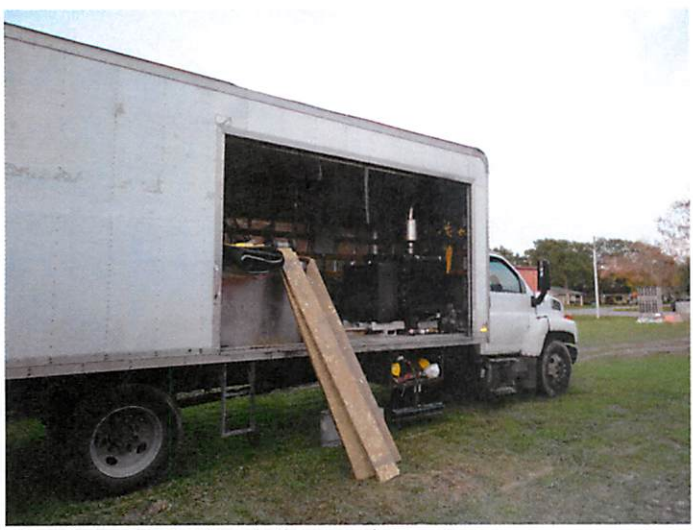
1. Spray foam insulation equipment
