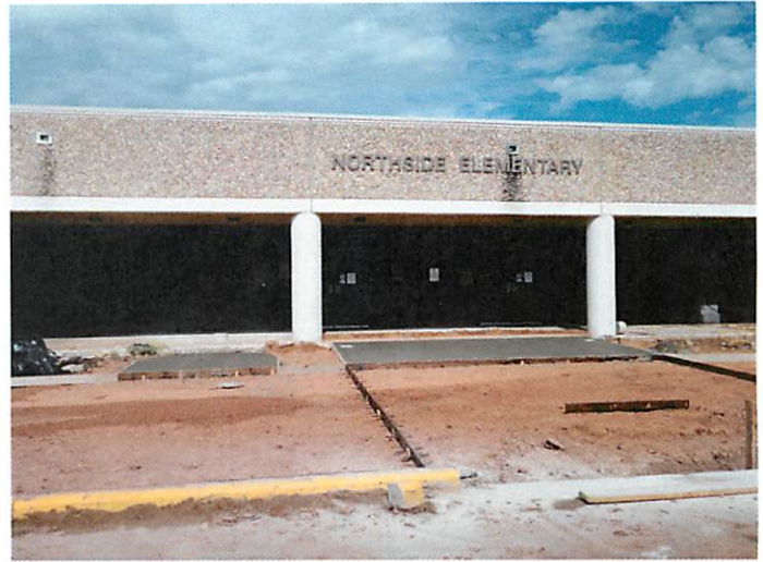
2. Northside Elem. – Concrete walks at front entry
