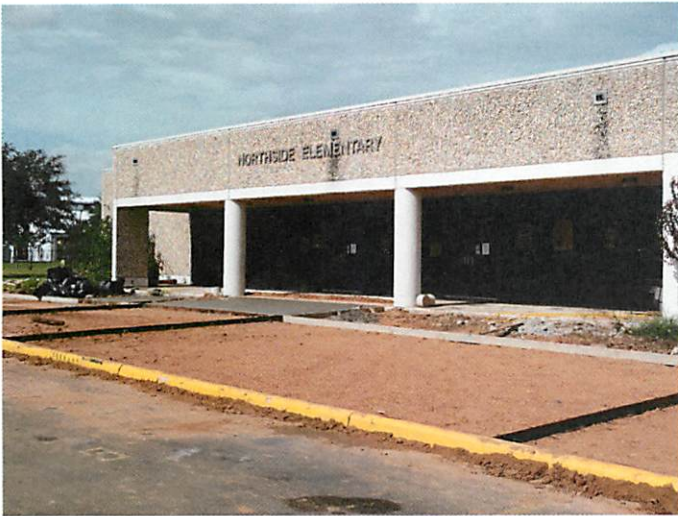
1. Northside Elem. – Concrete walks at front entry
