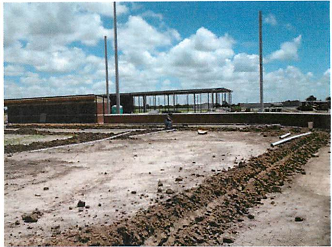
8. Irrigation system at baseball field
