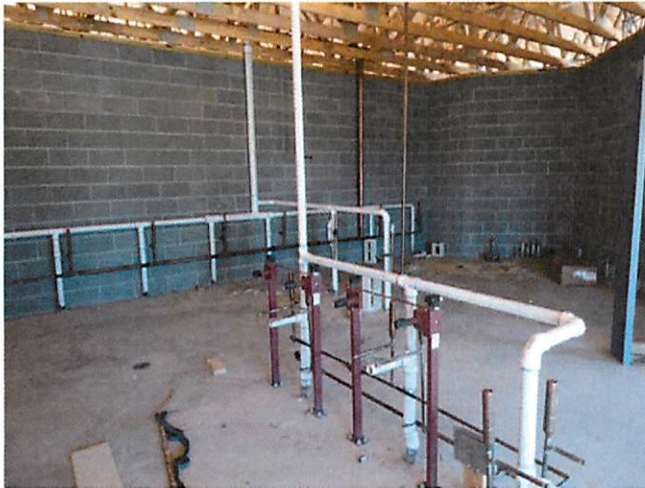
9. Plumbing vent / water at concession building
