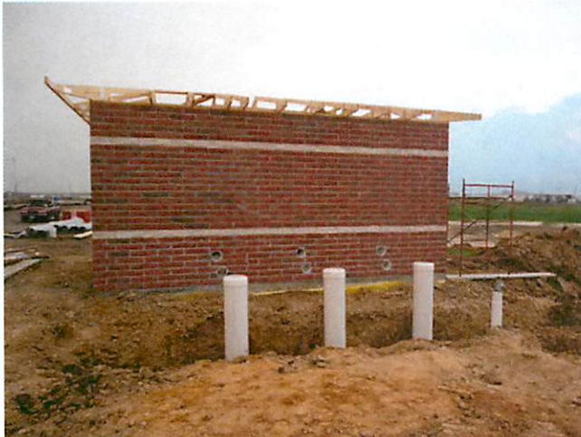
9. Wet well piping at irrigation building
