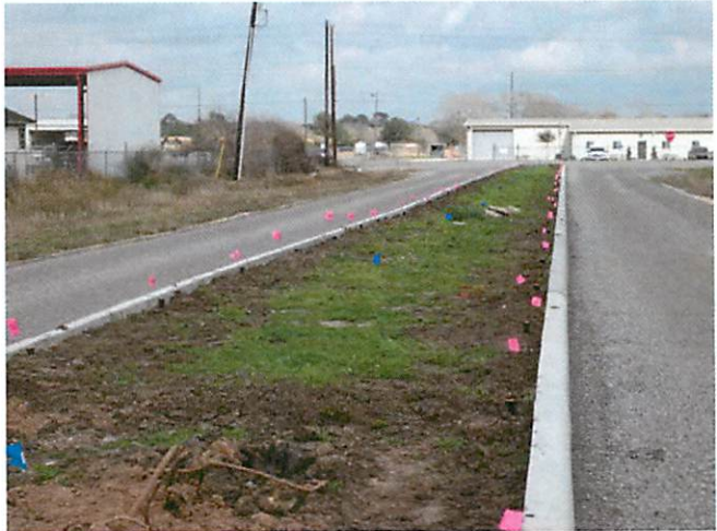
8. Irrigation system at main drive
