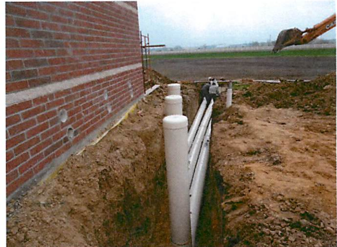
10. Wet well piping at irrigation building
