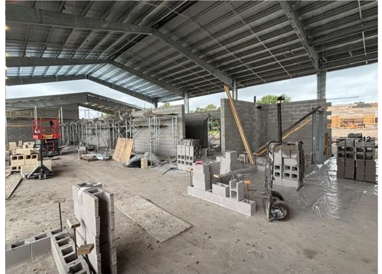
CMU Block being laid at the pins, feed, and storage area – Show Arena
