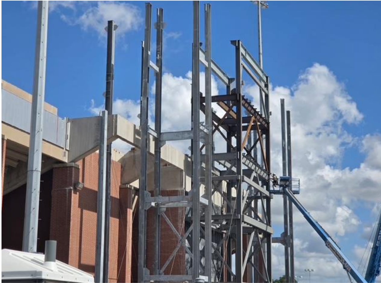
Detailing of the structural steel system for the new press box is underway
