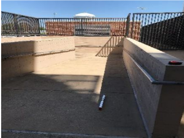
Ramps not ADA compliant
