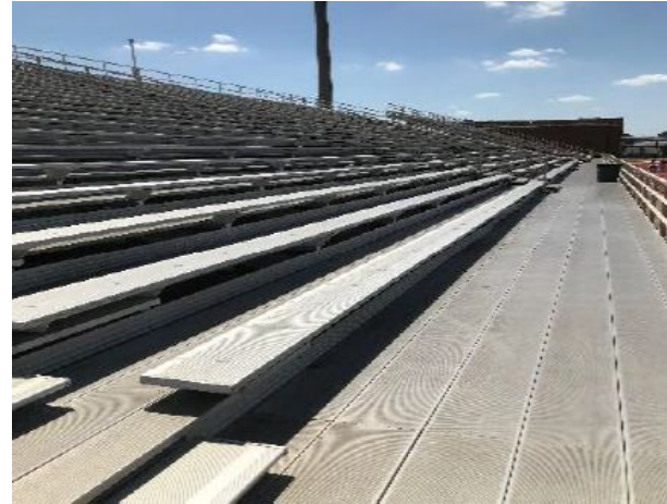
No ADA access to stands or ADA seating at front of stadiums.
