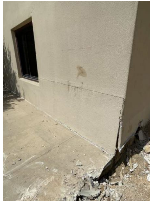
Deteriorated stucco wall system
