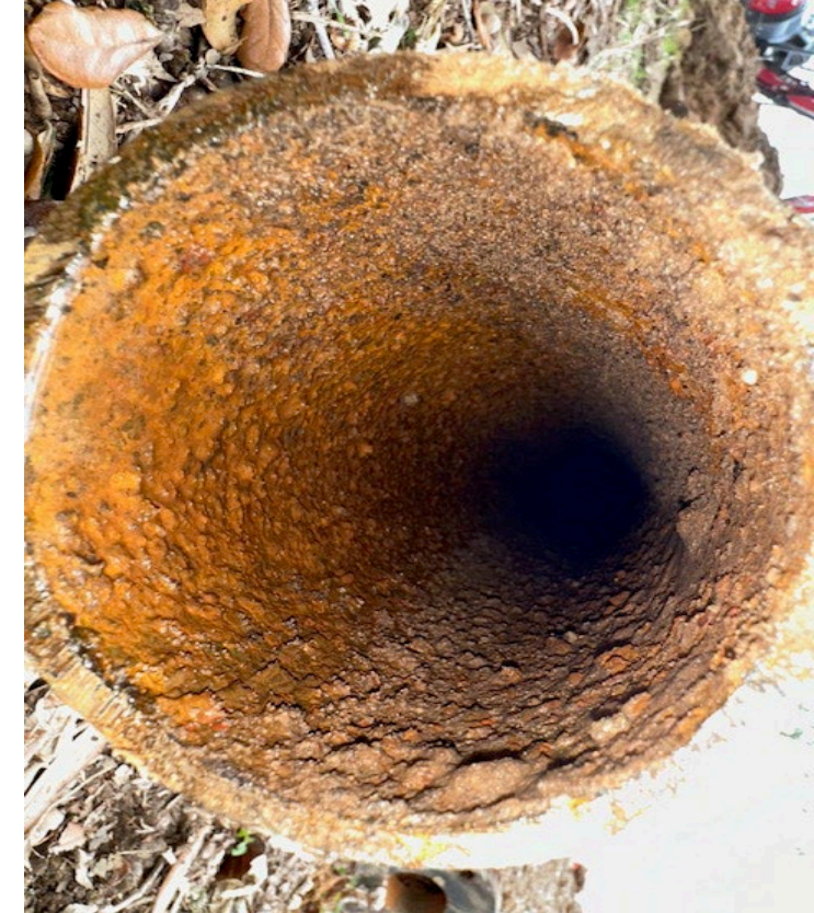
INTERIOR RUST DETERIORATION
