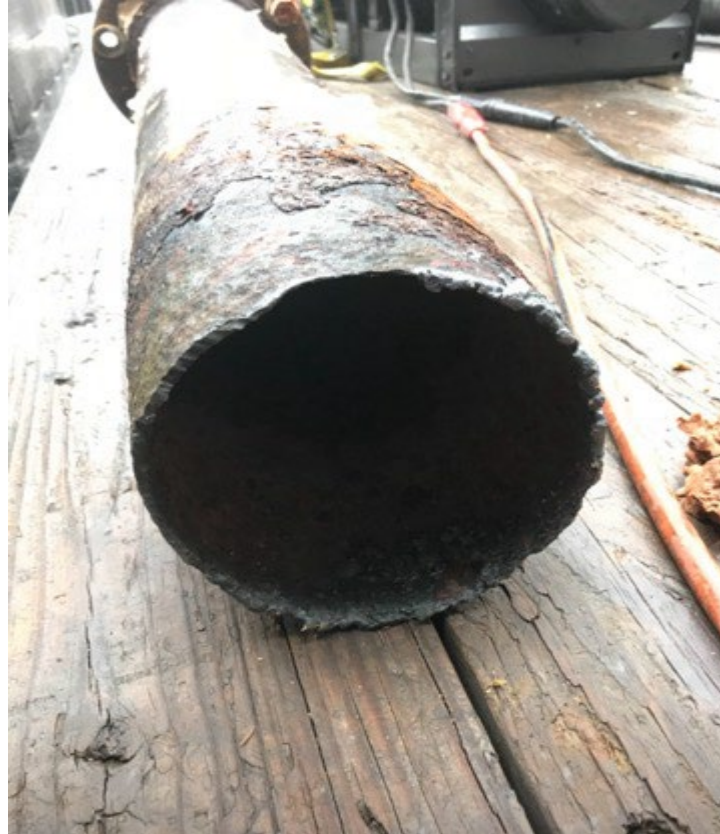
EXTERIOR RUST DETERIORATION
