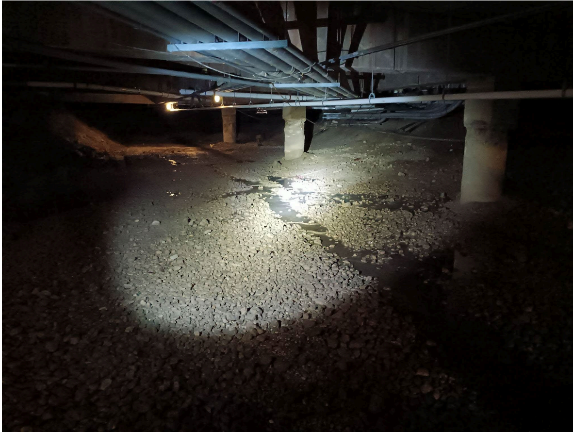
UNDERFLOOR ELECTRICAL BUS
