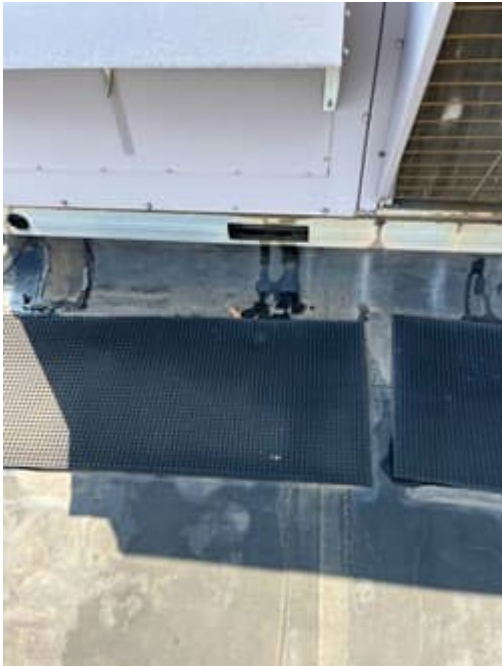
AC Unit is leaking
