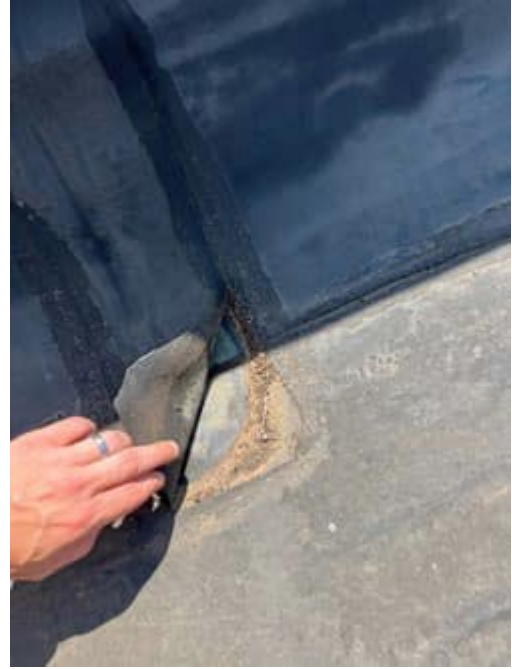
Exposed seam on parapet
