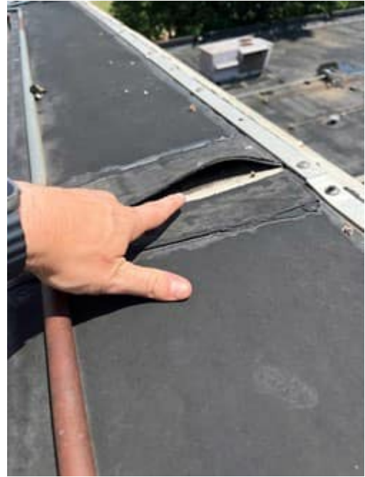
Open seam along coping
