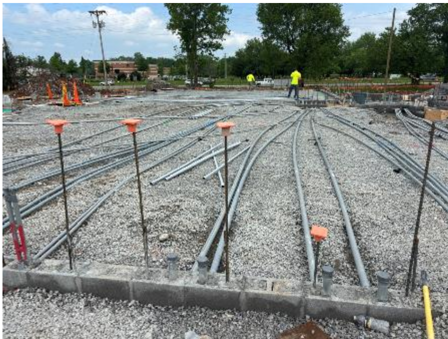
Under Slab Utilities
