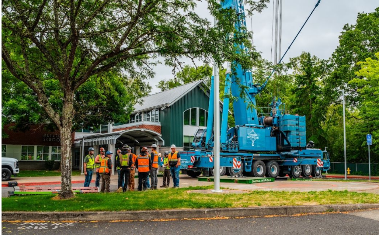
Metzger Elementary General Contractor - Piper Mechanical
