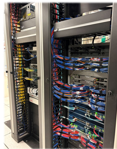
Data Center Rack (RWAN)
