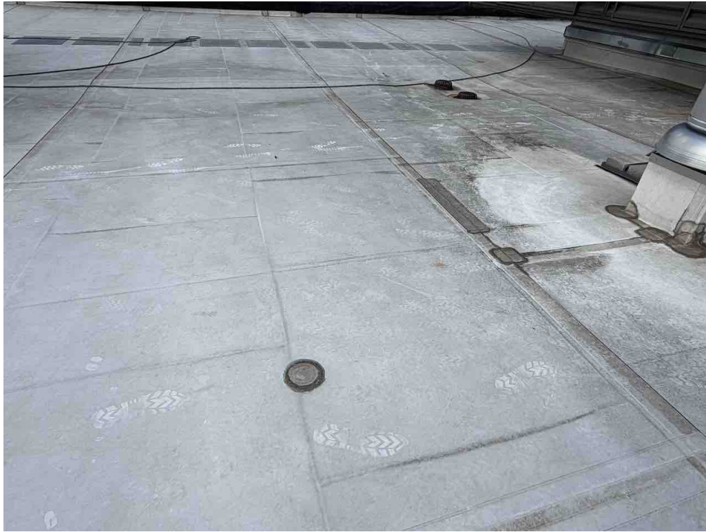
#27 -- Section A: Overview showing membrane patches. [2601301R0027.jpg]
