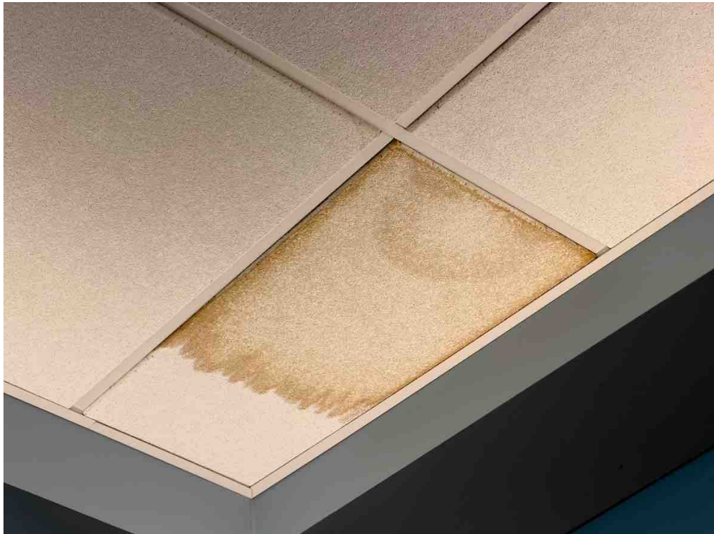
#2 -- Section INT: Close-up showing stained ceiling tile in Leak Area #1. [2601301R0002.jpg]
