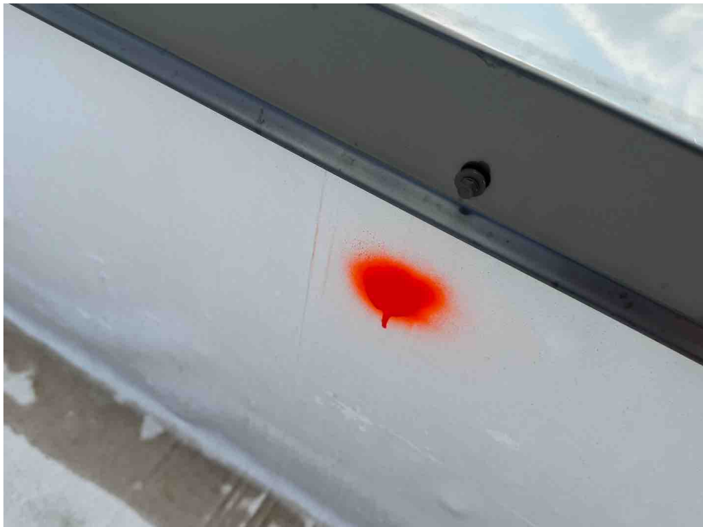
#18 -- Section A: Close-up showing a loose fastener on the perimeter metal coping. [2601301R0018.jpg]
