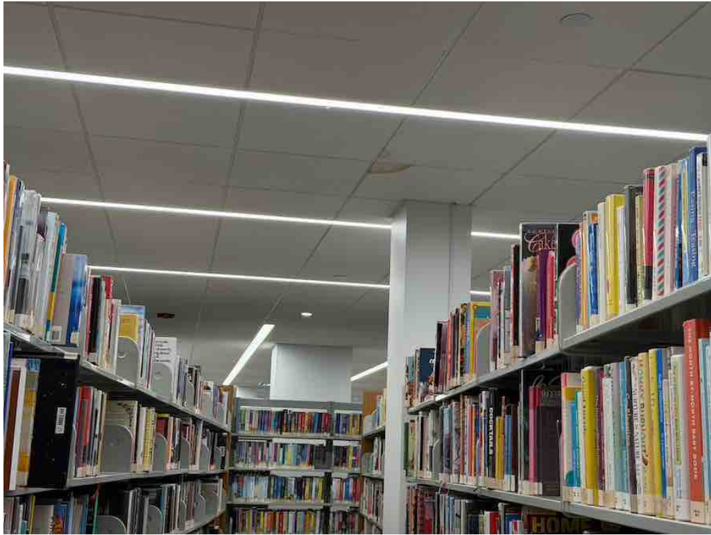
#3 -- Section INT: Overview showing stained ceiling tile in Leak Area #2. [2601301R0003.jpg]
