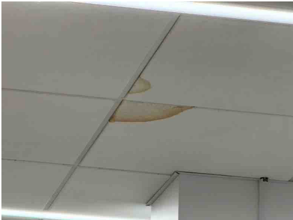
#4 -- Section INT: Close-up showing stained ceiling tile in Leak Area #2. [2601301R0004.jpg]
