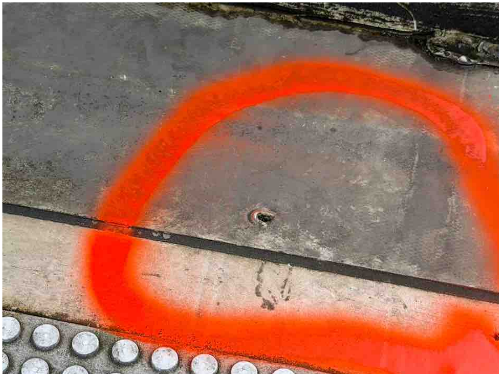
#12 -- Section A: Close-up showing a gouge/hole in the roof membrane. [2601301R0012.jpg]
