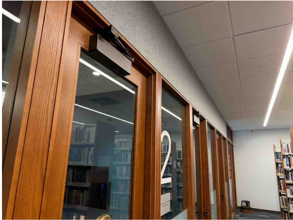
#5 -- Section INT: Overview showing Leak Area #3. [2601301R0005.jpg]
