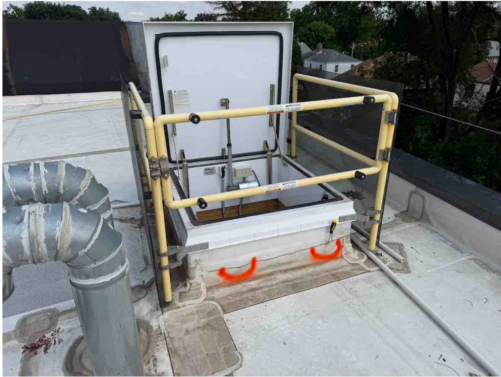
#9 -- Section A: Overview showing roof hatch flashing open at the top. [2601301R0009.jpg]
