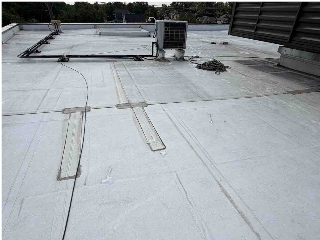
#26 -- Section A: Overview showing membrane patches and small air blisters. [2601301R0026.jpg]
