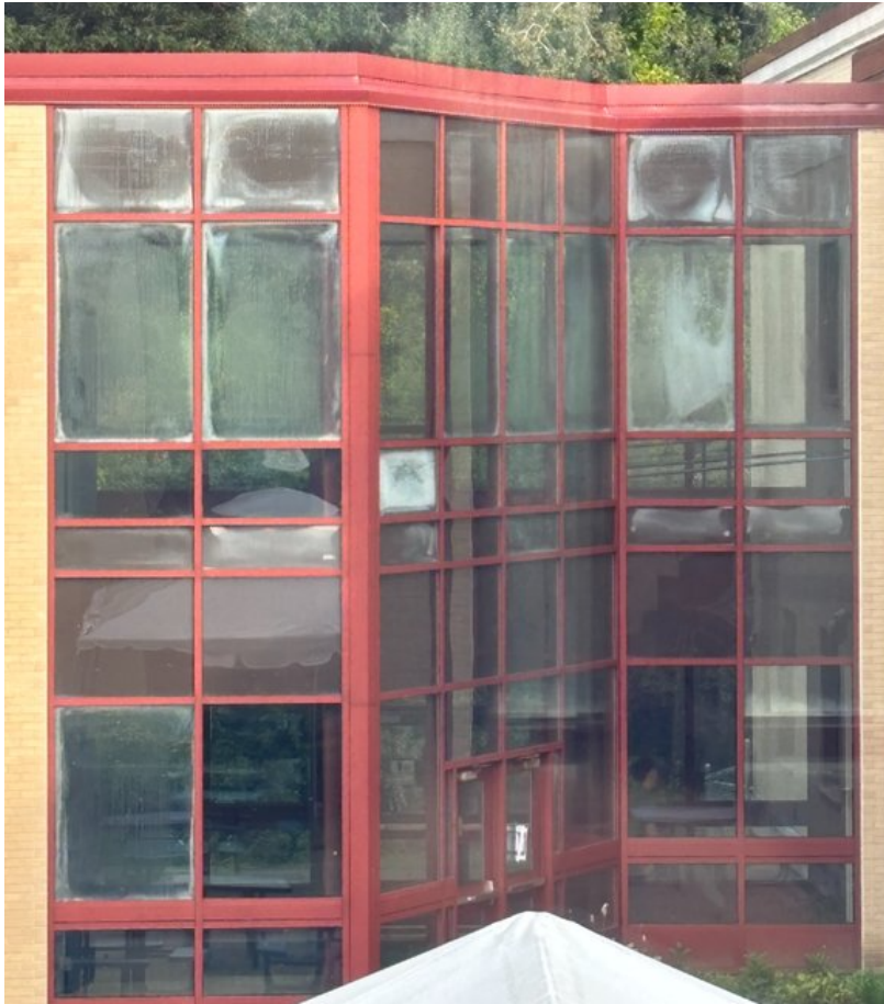
Example of failed insulated glass
