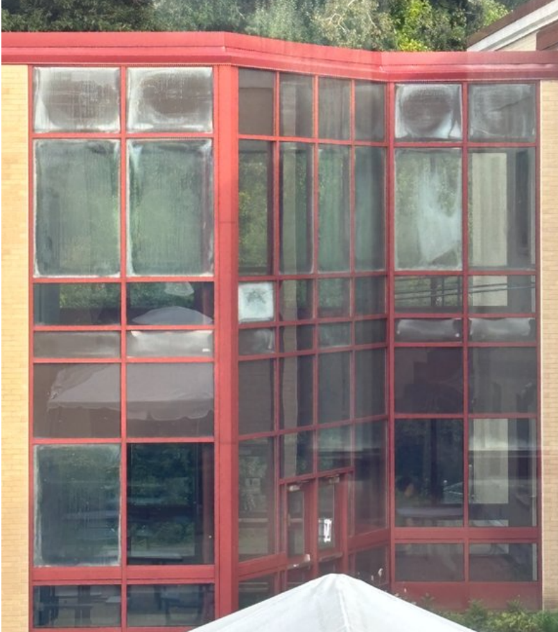
Example of failed insulated glass
