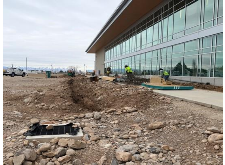
Lighting installation around Performing Arts
