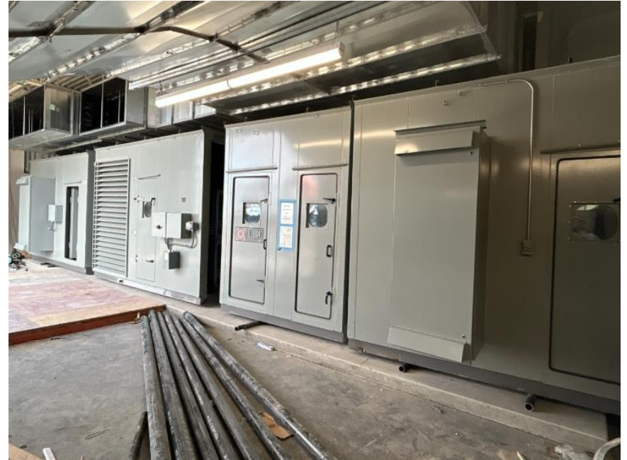
Air handler located in Mechanical Room
