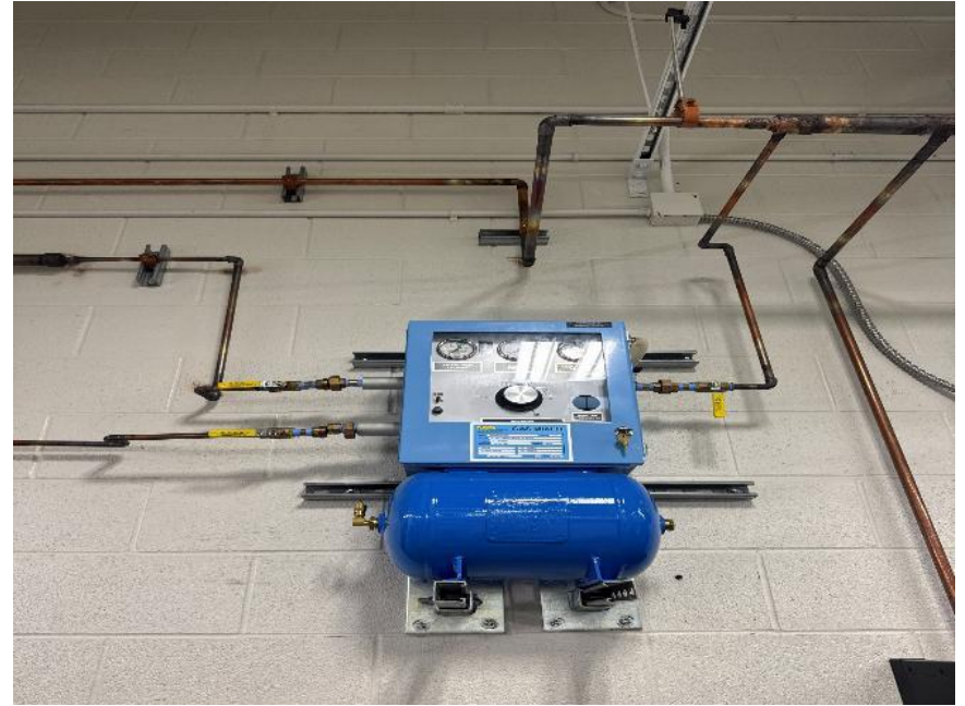
Carbon dioxide in argon mixer for Welding Shop
