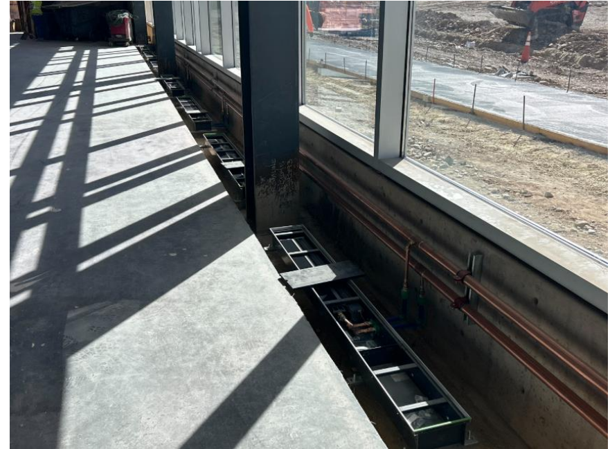
Auditorium lobby radiant heat floor system
