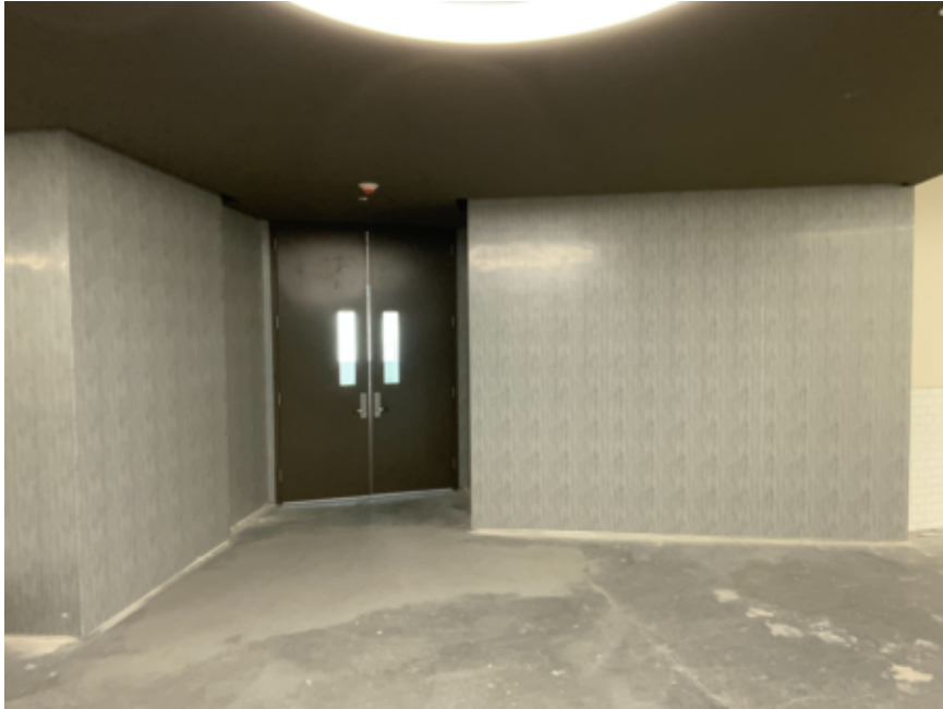
Impact resistant wall paneling on Level 3
