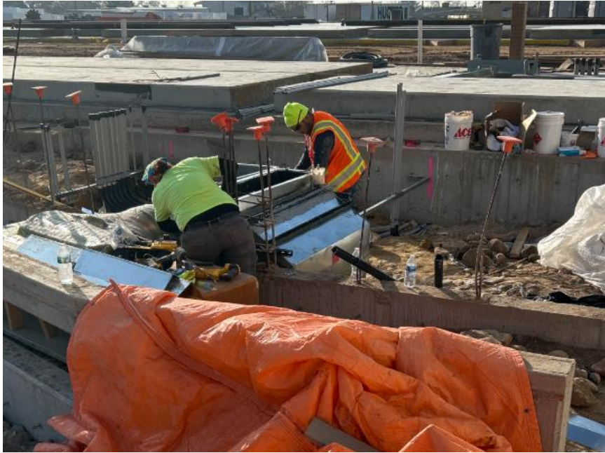
Underground HVAC west of the Auditorium
