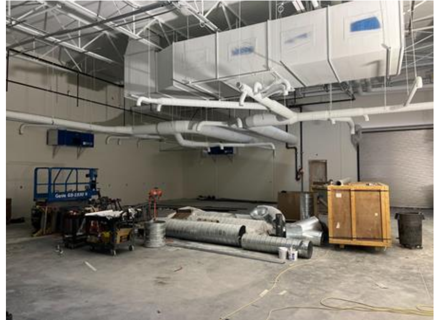
Fire protection in the Manufacturing Shop
