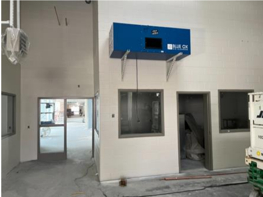
Air filtration in the Manufacturing Shop
