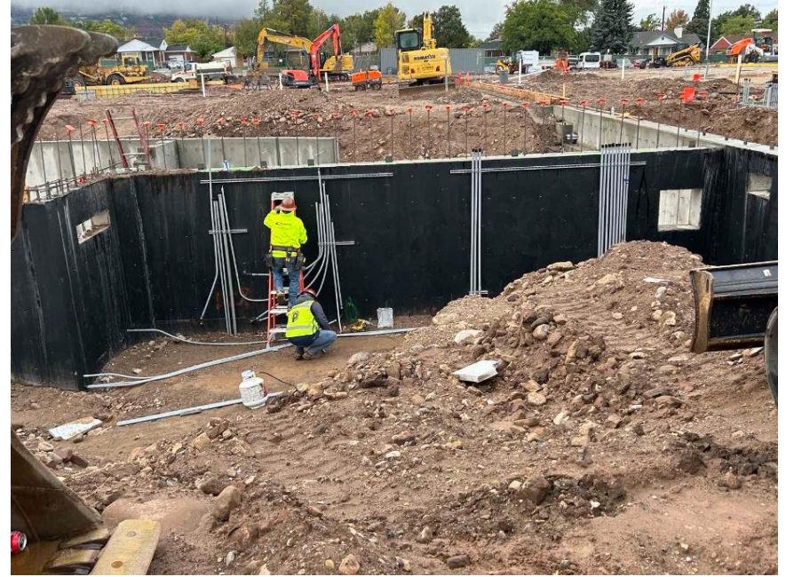
Electrical conduits north of the orchestra pit
