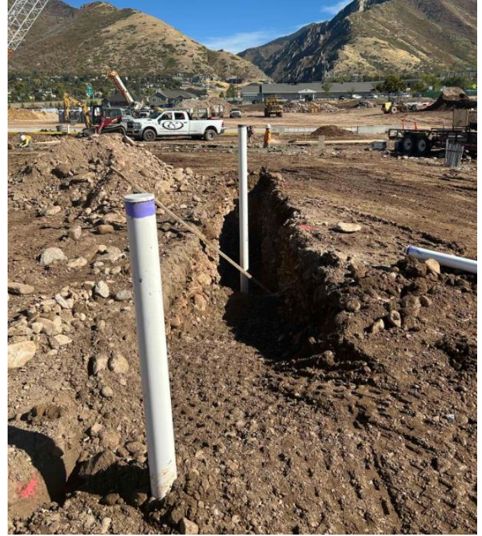
Plumbing installation south of the orchestra pit
