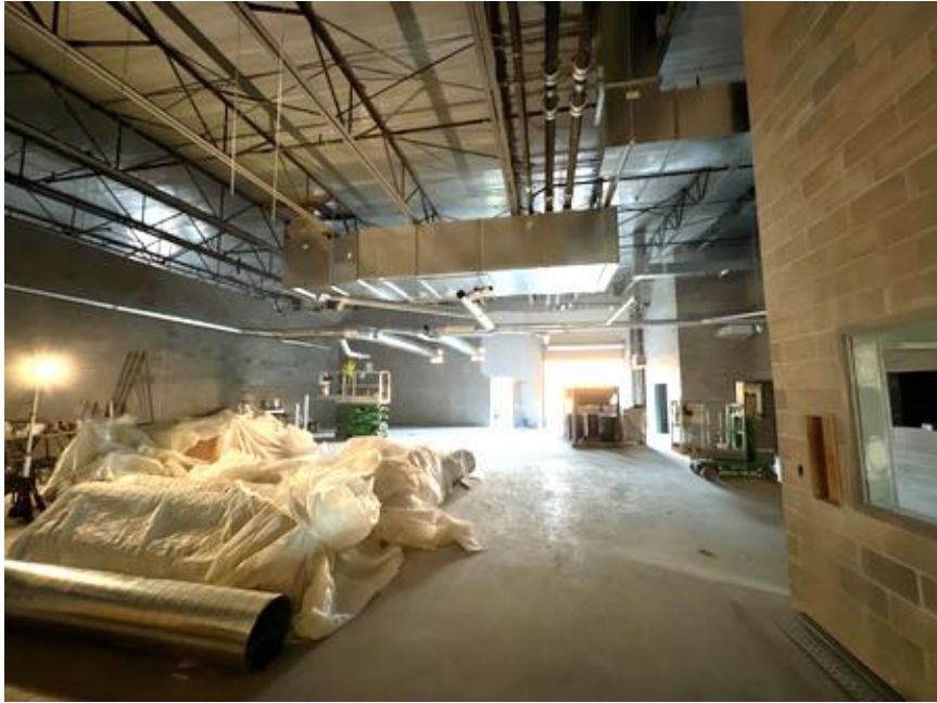
HVAC in Manufacturing Lab
