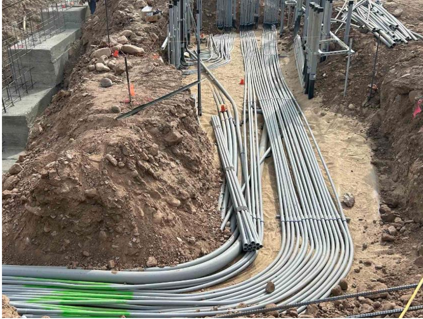
Electrical conduits east of the orchestra pit
