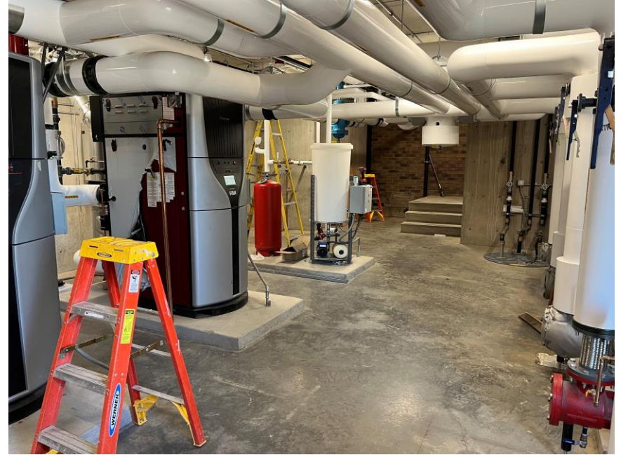
Central Plant interior
