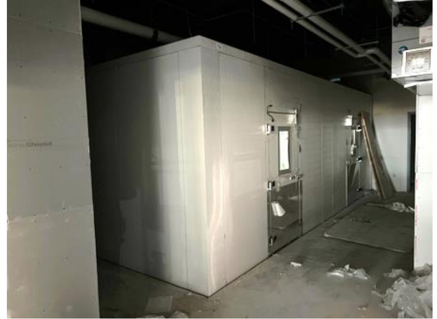
Walk in freezer in the Kitchen
