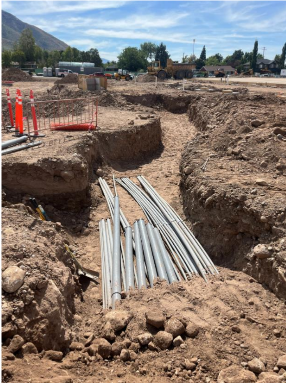
Underground electrical conduit running along the west side of the Orchestra pit
