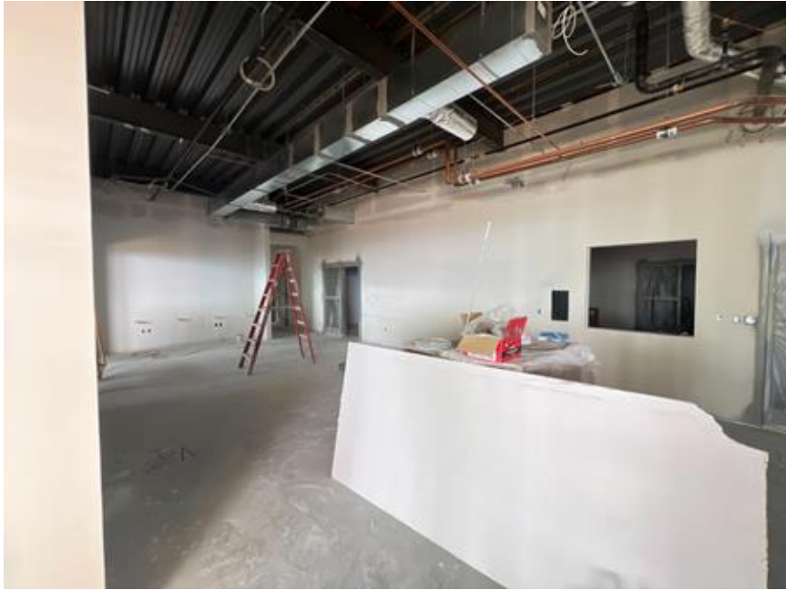
Paint on Level 1 of Administration
