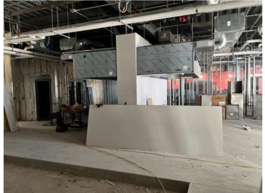
Commercial hoods in the Kitchen
