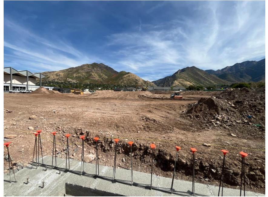
East parking lot being prepped. Majority of dirt haul off is complete
