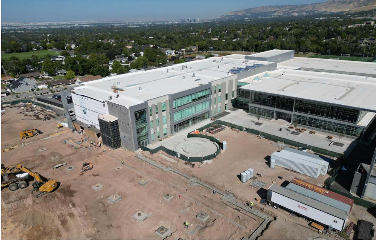
New Academics building with student courtyards. New Performing Arts building 30 footings at bottom of picture
