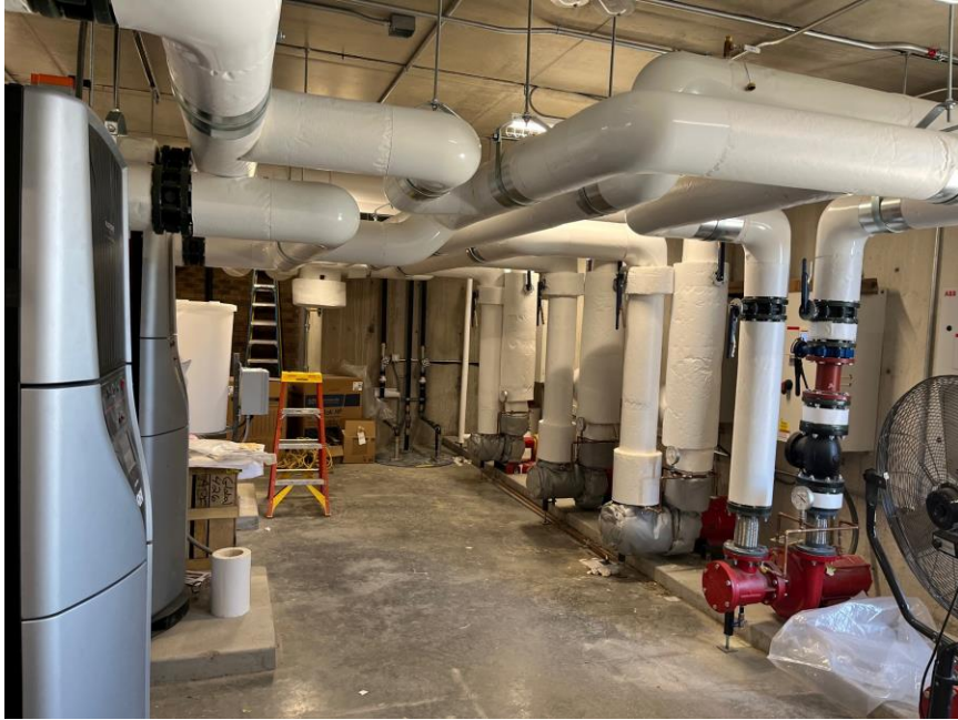
Central Plant Interior
