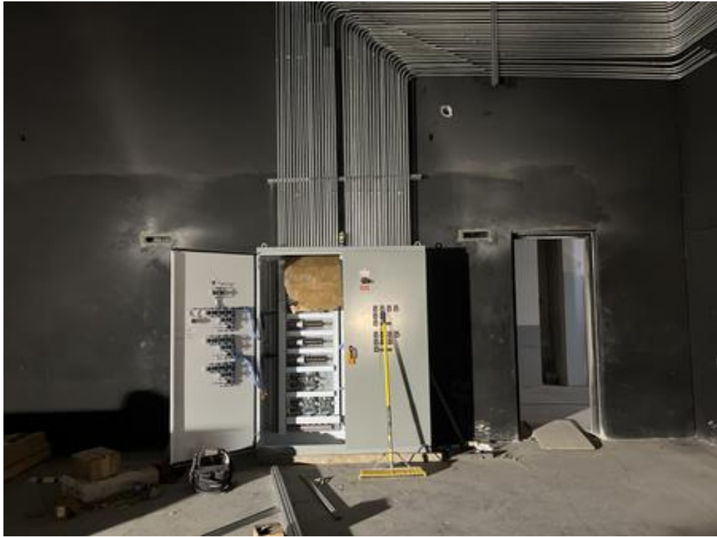
Stage motorized rigging
