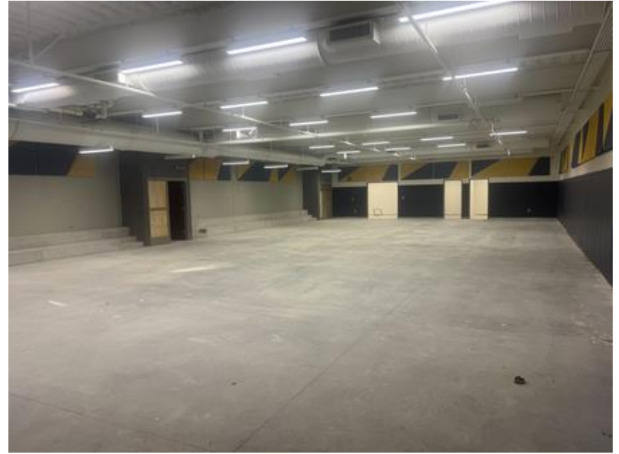
Permanent lighting in Wrestling Room
