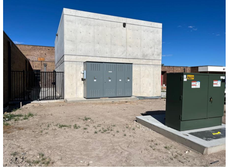
Central Plant Exterior
