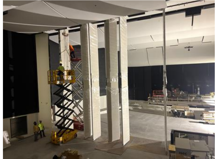
Operable partition in the Auditorium
