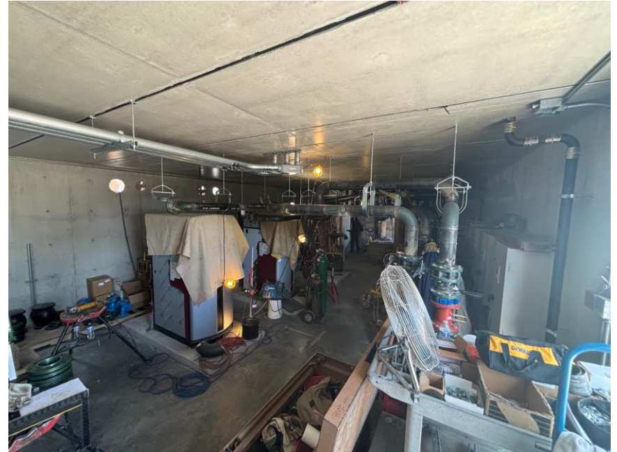
Interior of the Mechanical Room
