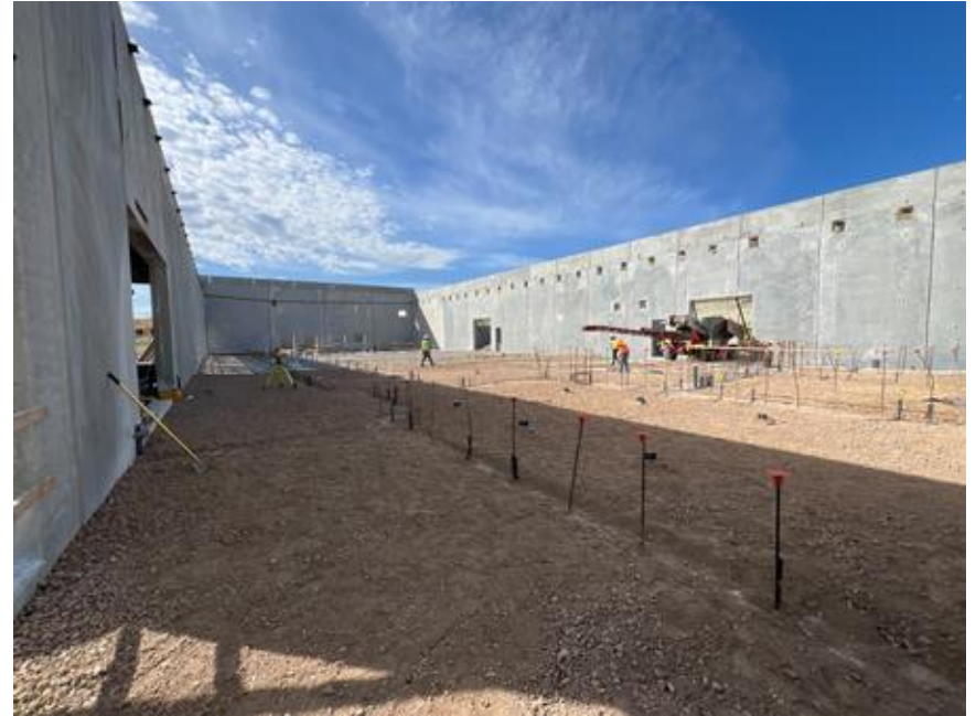
Manufacturing Shop plumbing/electrical
