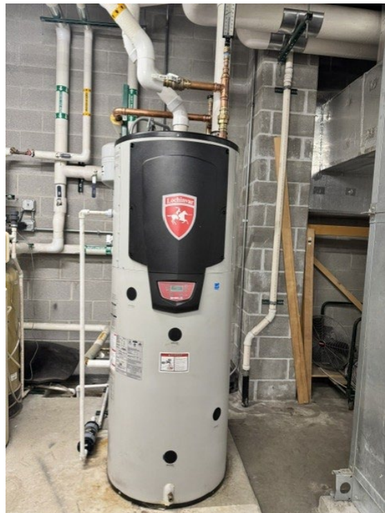
New hot water tank installed.
