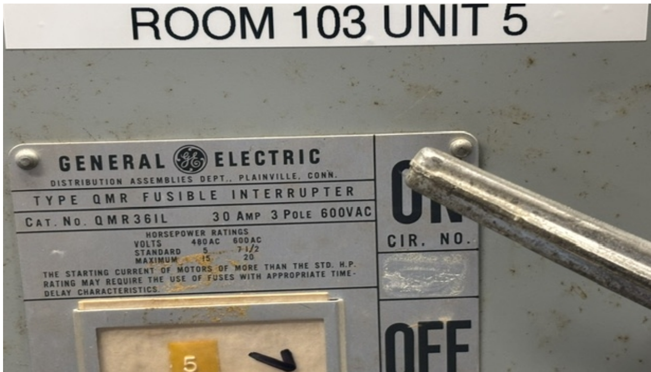
Electrical Panel Information
