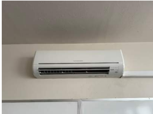
Figure 8 Split-system AC units serve the IT office and server room to provide cooling.
