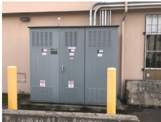
Figure 12 Existing Electrical Service #1 (MSP)
