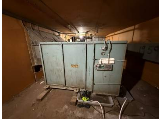
Figure 6 The gym air handling unit has steam heating coils and while currently functional, is past end of useful life.
