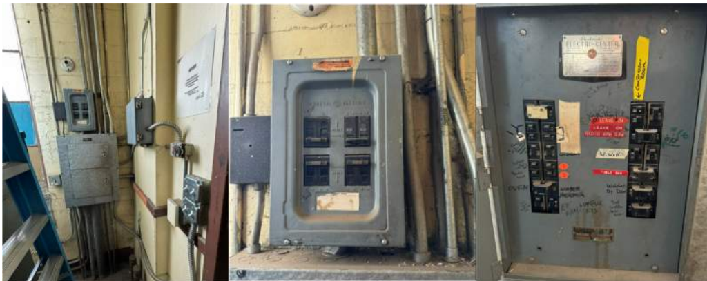
Figure 20 Load centers in existing Shop Building
