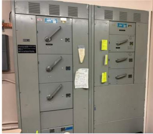
Figure 17 Existing Electrical Service #3
