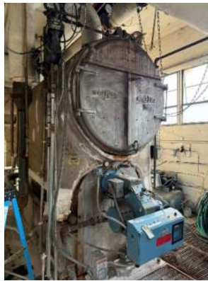
Figure 5 The existing steam boiler is aging and minimally functional. Steam distribution throughout the building is failing and sections of piping have had to be valved off to prevent leaks coming up through flooring.
