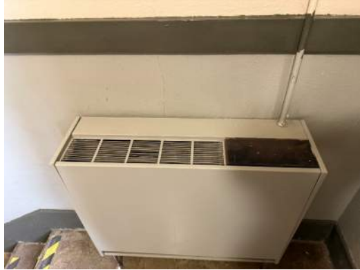
Figure 7 The unit ventilators serving the admin building are not functional and past end of useful life.
