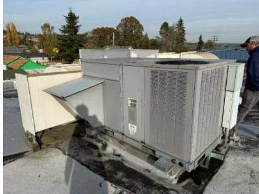
Figure 2 There are four rooftop air handling units that past expected useful life.
