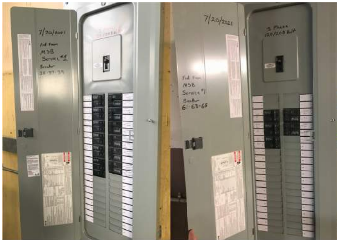
Figure 19 Branch Panels W and M fed from MSP in existing Shop Building
