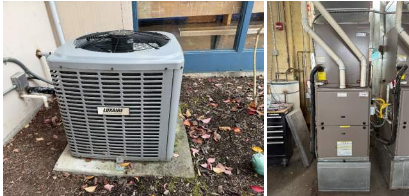
Figure 3 The classrooms are served by residential style furnaces and outdoor condensing units.
