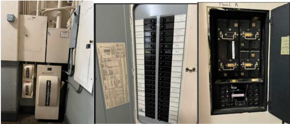
Figure 18 District Office Panels and Disconnects
