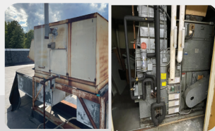
Aging Mechanical Systems: Mechanical systems are at their end of useful life
