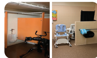
Inadequate Restrooms: Restrooms are small, difficult for mobility devices, and not adjacent to classrooms
