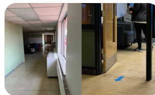
Mobility Obstacles: Narrow hallways and common areas hinder accessibility and observation
