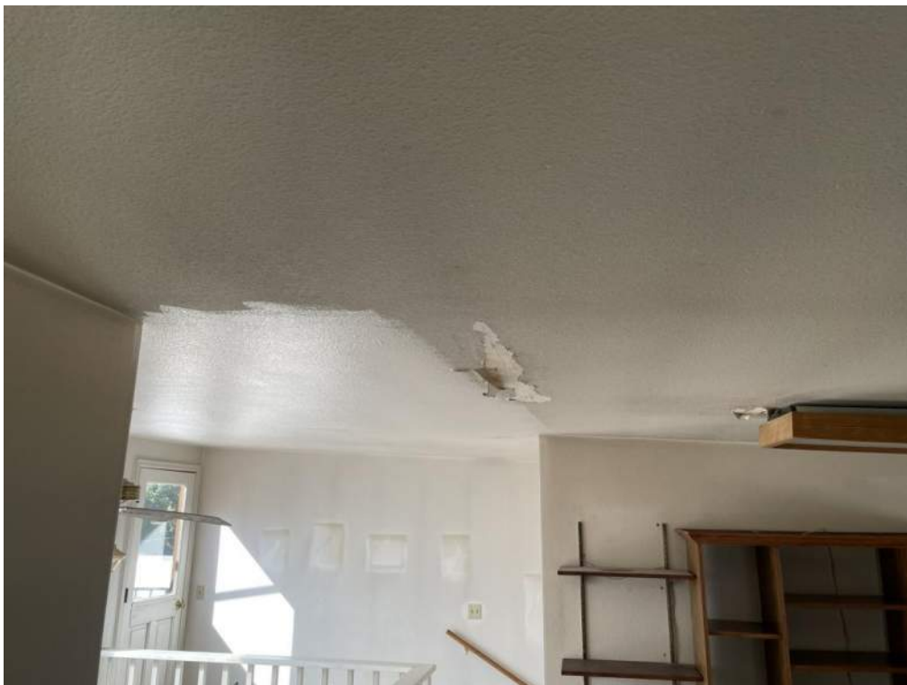
Figure 6- Damage to third floor ceiling.
