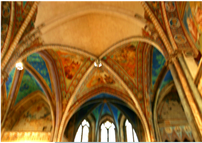
Polymeric resins, Glass, Carbon and Aramid Fabrics were used in repairs for earthquake damage.
