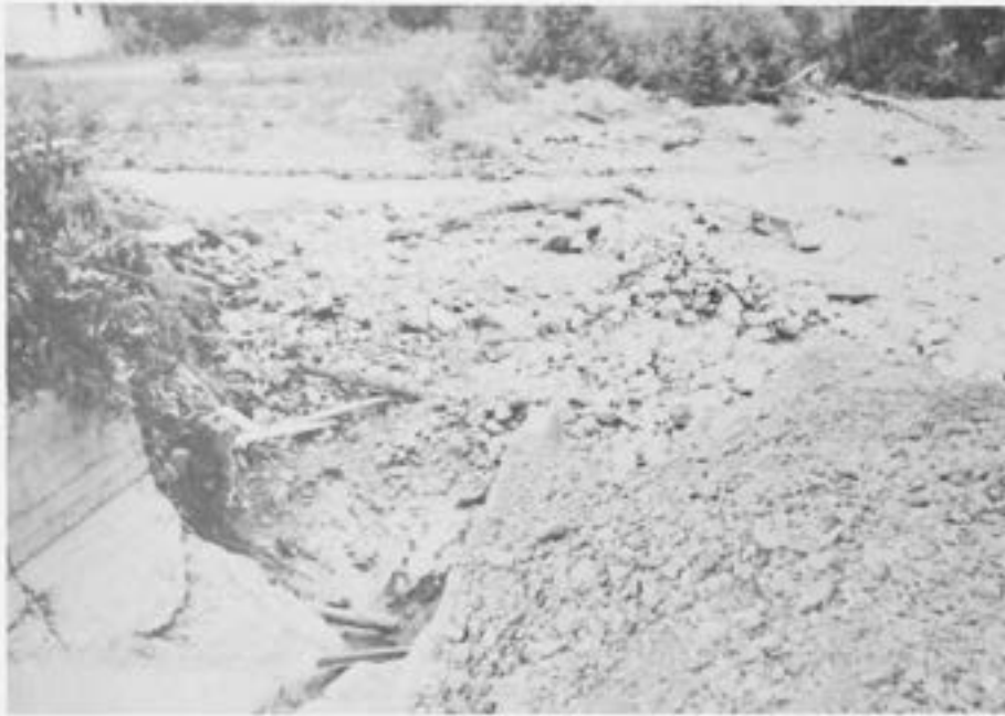
Figure 36. Debris accumulated at mouth of Portland Creek flume after 1982 event. (Photo courtesy William P. Stanton, CWCB)
